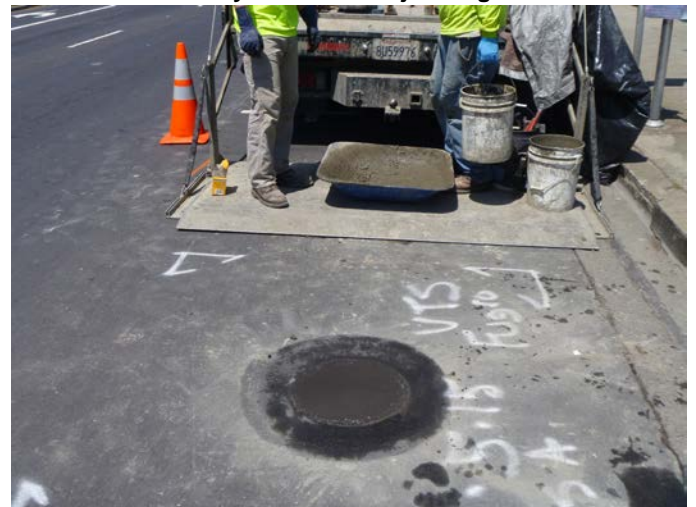
Monitoring wells patched with concrete and black dye to match adjacent grade
