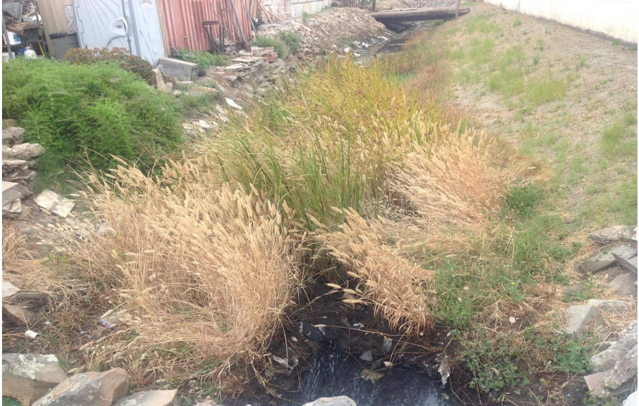
Photo 9: Drainage canal along western edge of site containing little to no water and wetland vegetation along the southern end of the canal within the site.
