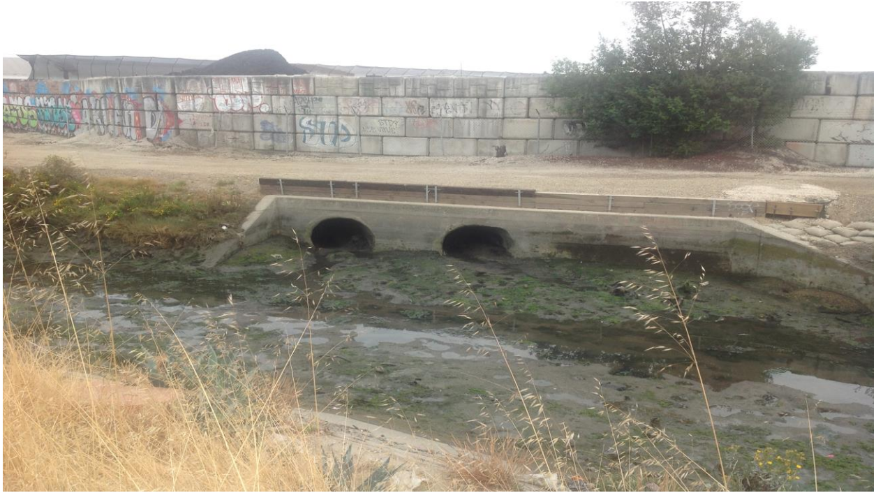
Photo 7: Storm water drain outlet within Seminary Creek coming south of the creek.
