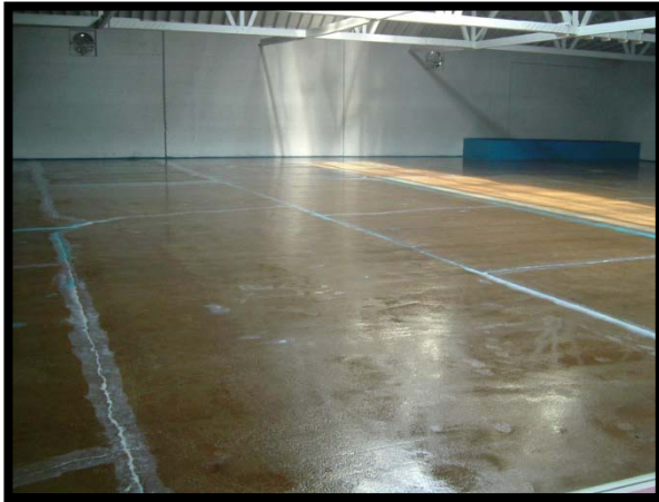
Completed surface preparation consisting of shot blasting, Retro-Coat PREP to fill joints and cracks and a 6 mil application of Retro-Coat PRIMER
