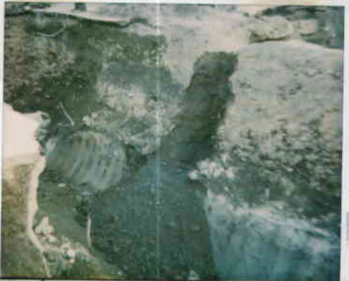
west flank of diesel UST pit - note discoloration
