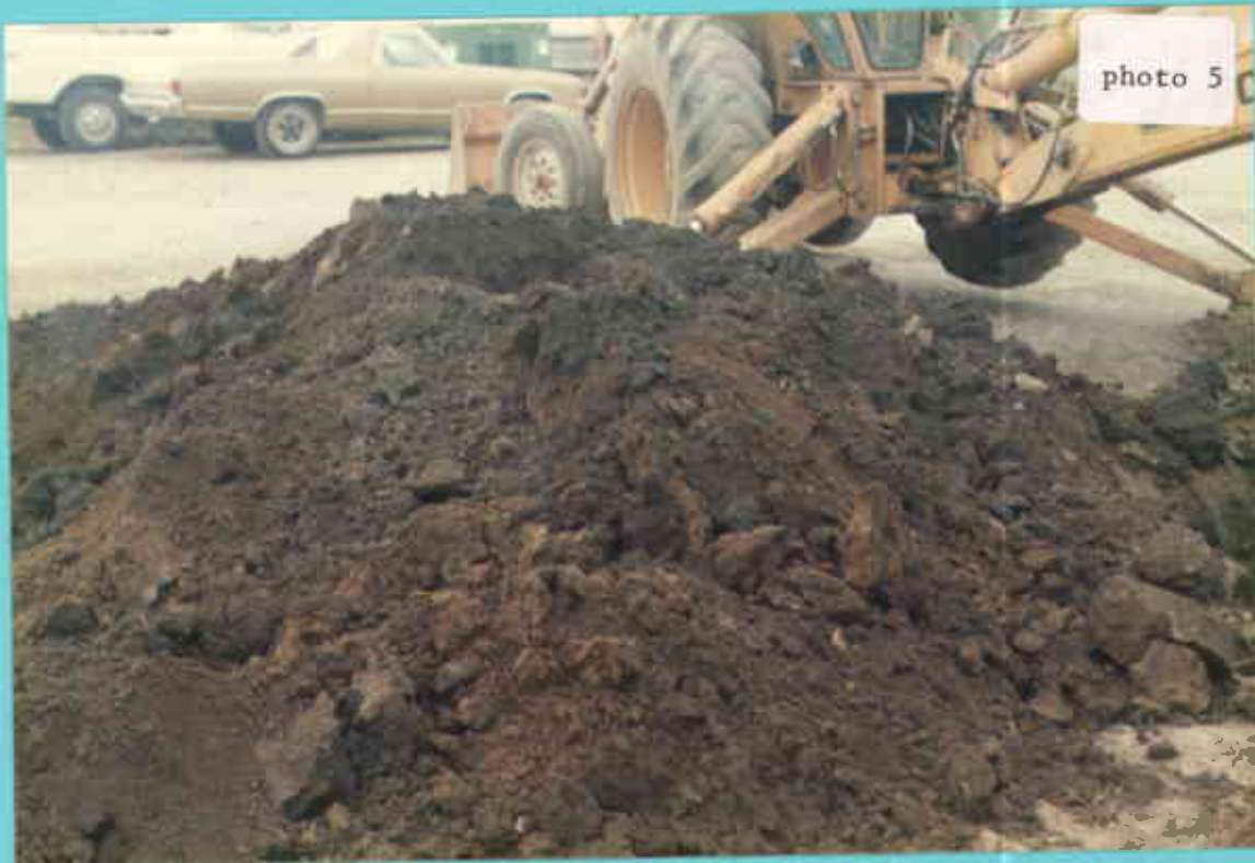
Photo 5. Mixture of contaminated soil and non-contaminated soil to be placed on treatment site.
