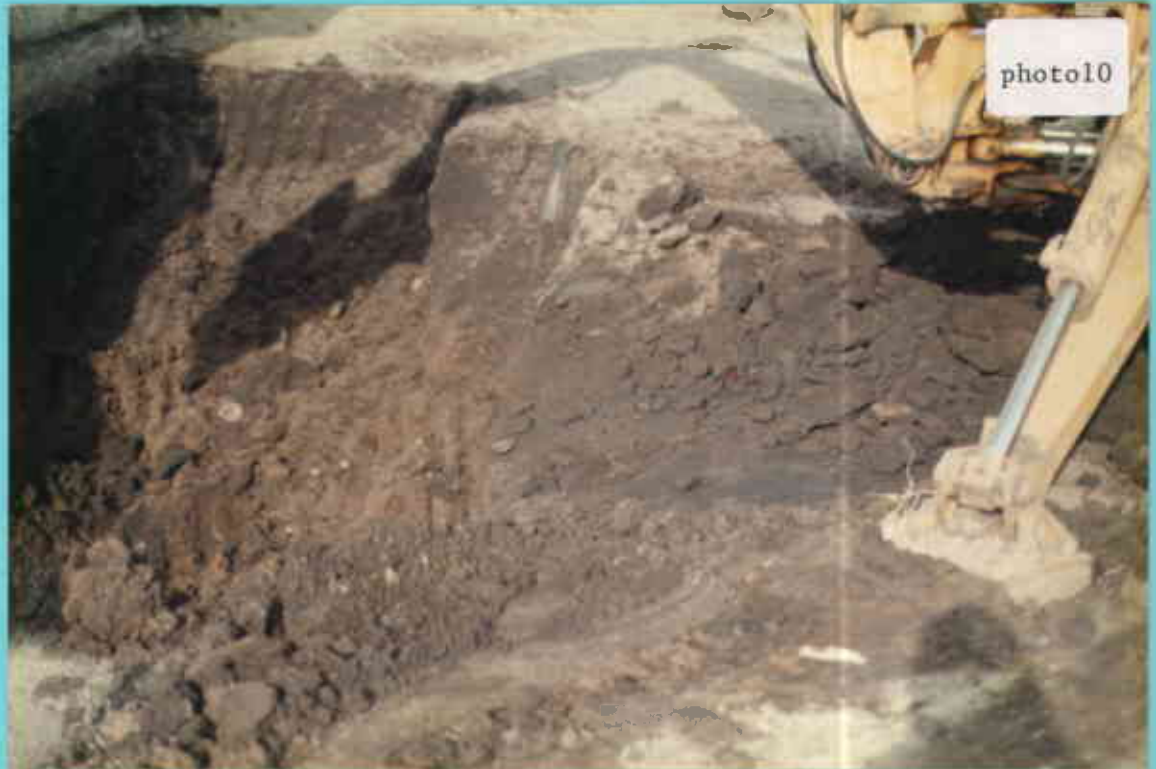
Photo 10. Exposed contaminated soil in southeast portion of the excavation.
