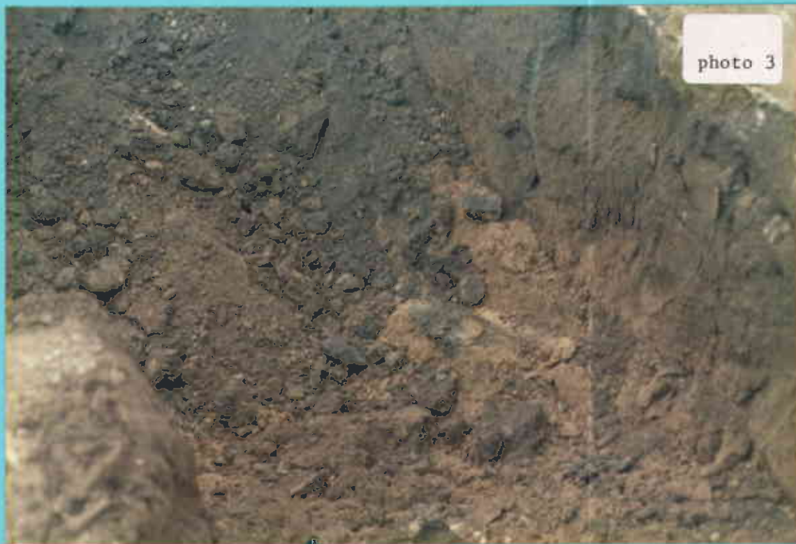
Photo 3. Bottom of excavation at north end showing light colored (uncontaminated) soils where conformation sample Sunol No. 5 was taken.
