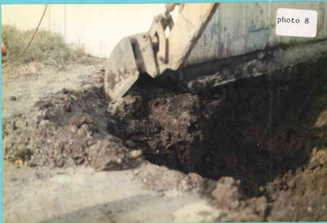
Photo 8. Excavation of material around the south east corner of the storage shed.
