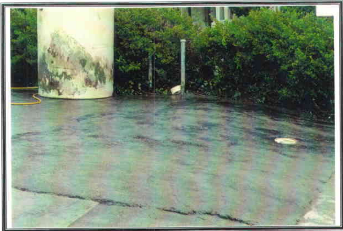
Photo No. 7- Temporary asphalt cover over the former excavation to protect the fill
