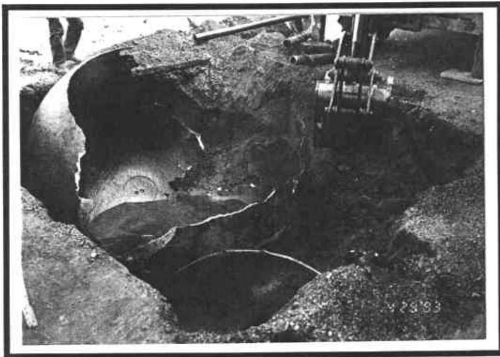
waste oil tank removal process - tank was broken into several pieces as a result of removal efforts
