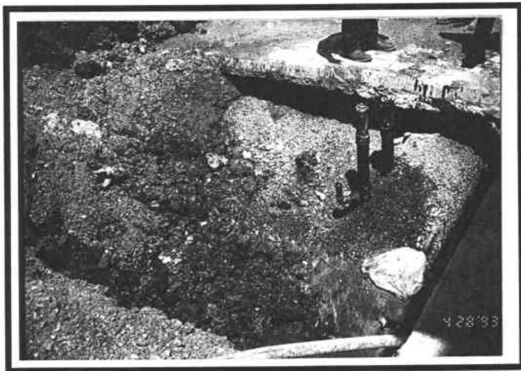
1,000 gallon bulk oil tank - punctured during excavation 4/28/93
