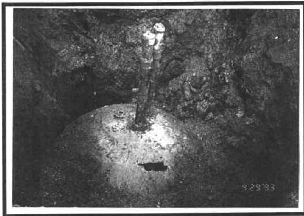
Bulk oil tank exposure with backhoe punctures in tank
