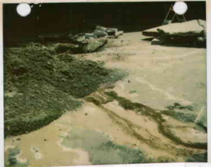
UPS 12215117976-8 4/28/93 8400 Pardee - W.O. tank pit W.O. leaching from stockpile
