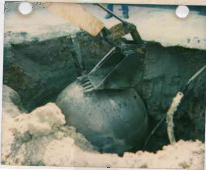
Fresh oil tank 12215117976-8 4/29/93 UPS
