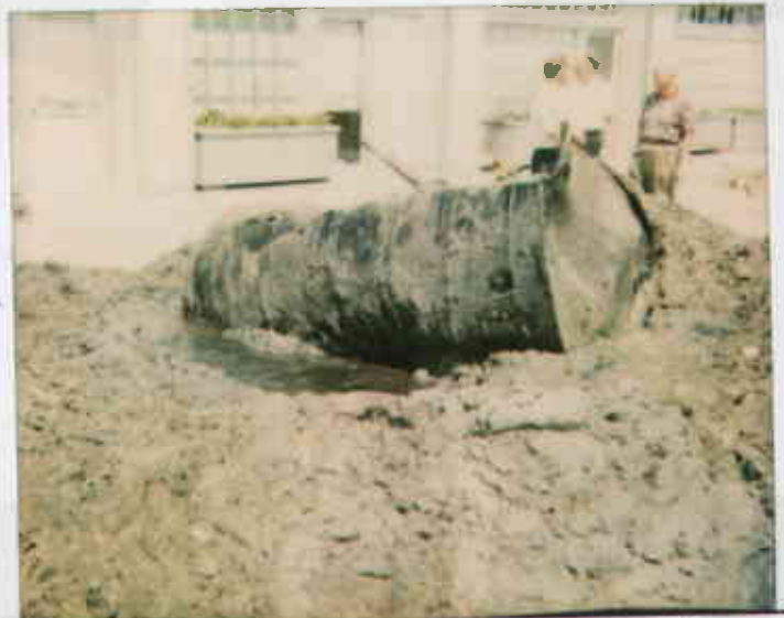
South UST ~500 gal - Corroded, w/ holes and drainage into stacked soil 8/6/97
