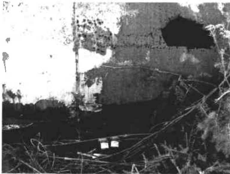
Photo no. 16: Sample CM05 was taken from this spot under tank T-1.
