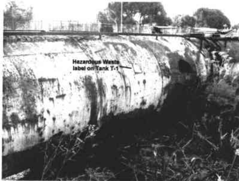
Photo no. 11: Tank T-1 had a worn out Hazardous Waste label on it.
