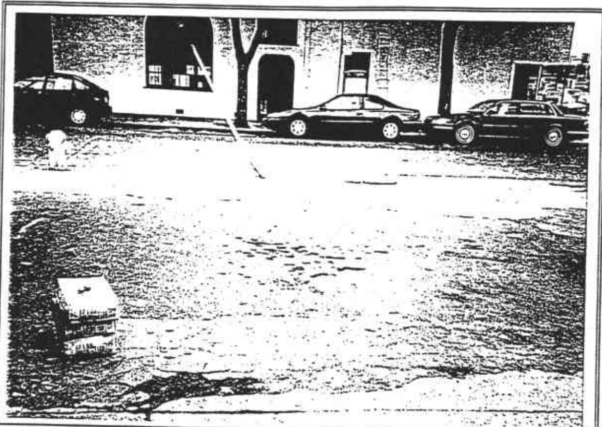
Photograph 7: Close-up view of the parking lot depicting the poor condition of the asphalt.
