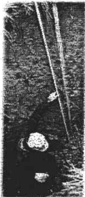
Excavation of a Geoprobe® Monitoring Well shows the quality annular seal around the well casing to a depth of about 10 feet bgs.
