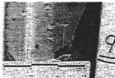
Close-up of the annular seal at 9 feet bgs. No voids in the grout and well casing remains centered in the annular space. (Blue scale in inches.)
