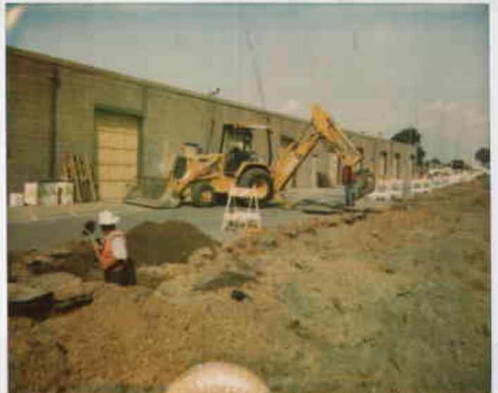
9/23/98 MSC south → north Phase I hydram lines being excavated 01717328093-2M 0026 5258 COPIES & ENLARGEMENTS CALL 800-421-1030
