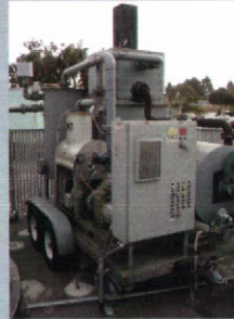
Dual-phase extraction & vapor abatement
