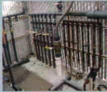
Piping to remediation wells
