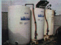
Activated carbon treatment
