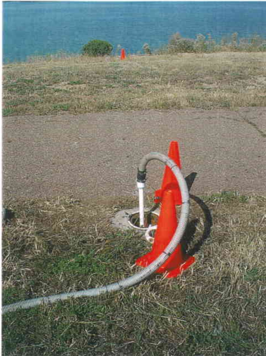
Photo 5: Dual-phase extraction from off-site Well MW-16.
