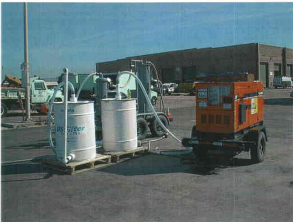
Photo 2: Activated carbon units for vapor control and electrical generator for the DPE system.
