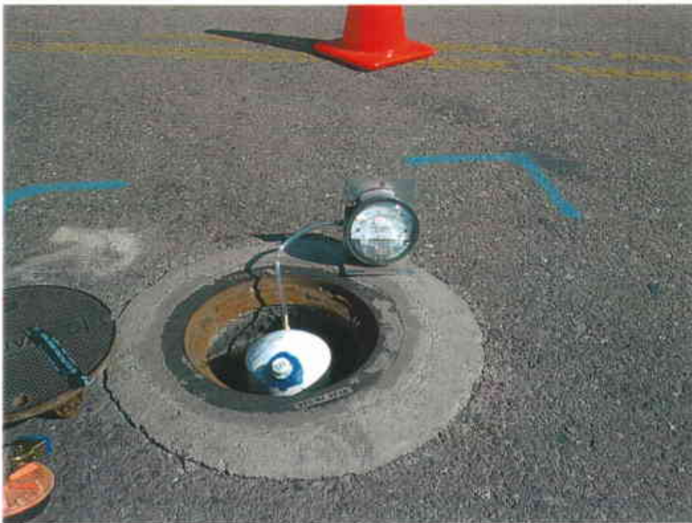
Photo 4: Monitor vacuum response from a monitoring well.
