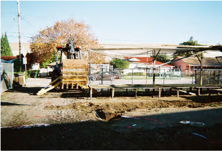
Photo 1 - View North. Excavation begins at the Lath House adjacent to groundwater monitor well MW-3. Backhoe bucket is 3 feet wide.
