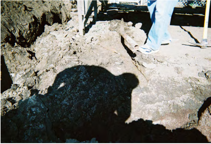
Photo 19 - View to the north of the cutoff metal water pipe.
