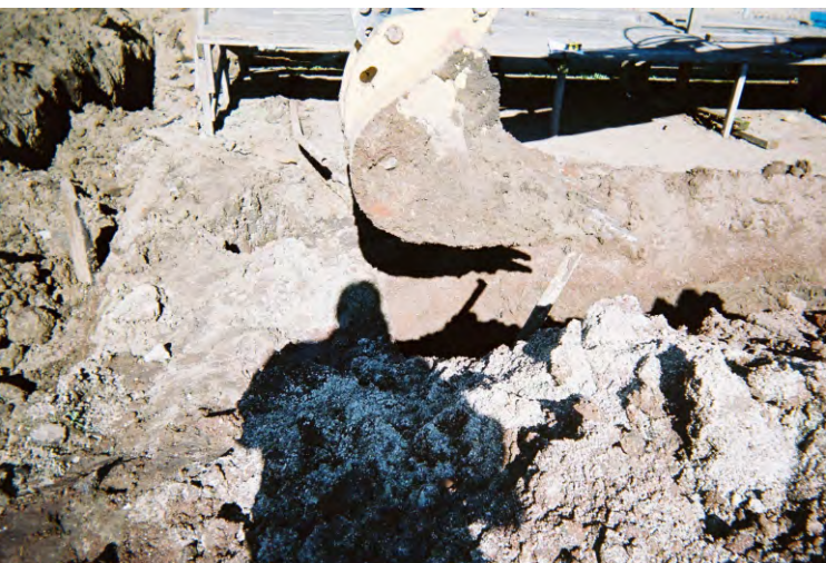
Photo 21 - View to the north of the east-west trending former gasoline UST pit showing the metal water pipe cut out over the trench.
