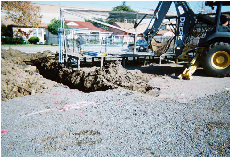
Photo 13 - View to the northeast of the termination of the south end of the north-south trending trench where a new trench was extended to the east at the suspected location of the former gasoline UST.
