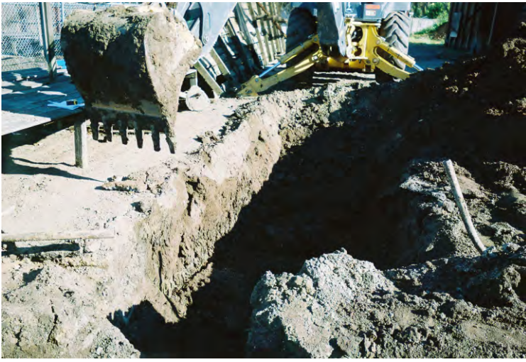
Photo 25 - View to the east along the former UST pit. The north wall of the trench shows the reddish fill soil to a depth of four feet bgs.
