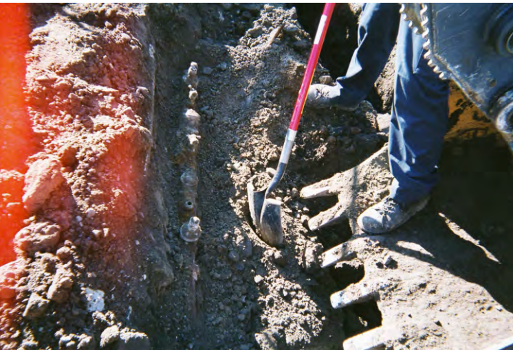
Photo 12 - View to the north of the north-south trending abandoned metal water line. This water line extends to the south and crossed over the top of the former gasoline UST, south of the fence line. This is very likely the cause of the magnetic anomaly identified to the north of the suspected former gasoline UST and north of the fence line.
