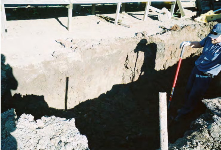
Photo 26 - View to the east along the former UST pit. After the fill, which was shown standing against the sidewall, caved into the bottom of the trench, natural black clay soil was now exposed in the side wall. It appears that the newly exposed side wall is the north wall of original gasoline UST removal pit.
