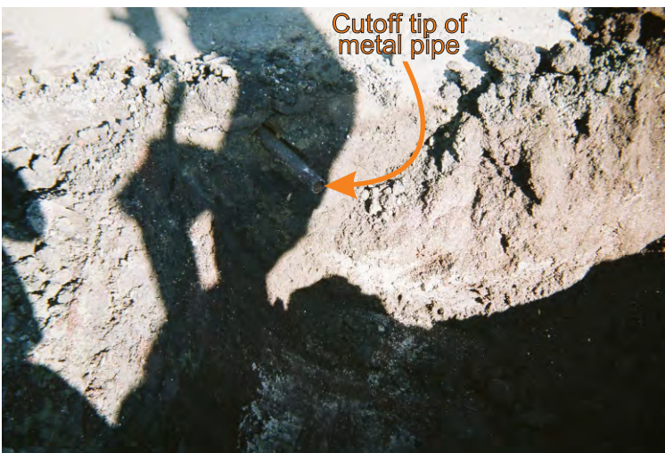
Photo 15 - View to the north of the former gasoline UST trench with cut off metal pipe sticking out of side wall. Notice the reddish colored vermiculite and crushed lava rock potting soil used as fill in the side wall.
