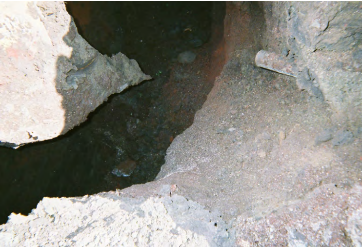
Photo 20 - View to the east of the east-west trending former gasoline UST pit with a cutoff metal water pipe sticking out of the south wall of the trench.
