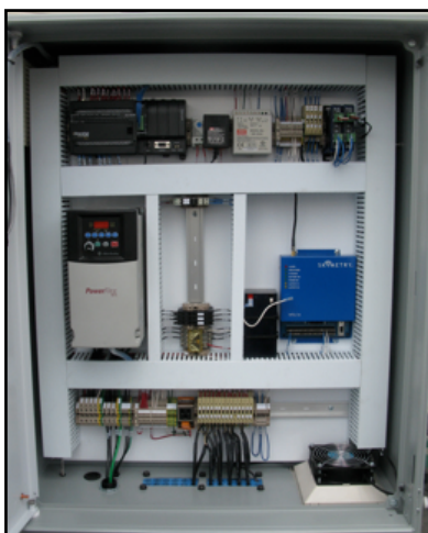
Control panel interior, shown with optional cellular dialer and VFD.
