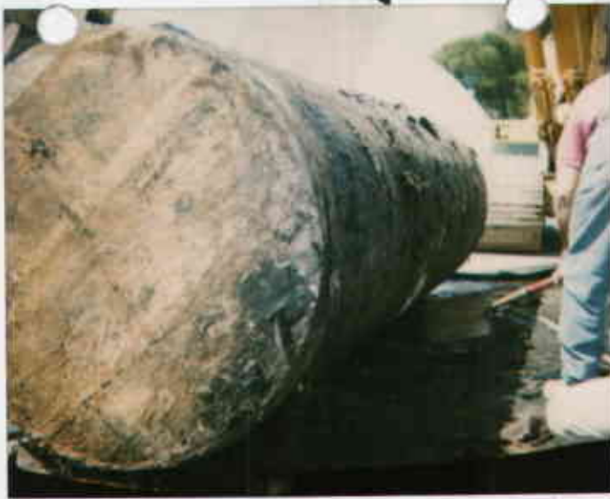
1000 gal gasoline UST
