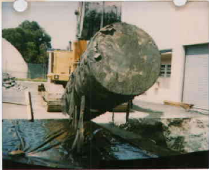
10000 gal gasoline UST 5/3/95 w/deteriorated tar wrap 0150, 2600 Grant Ave San Jo
