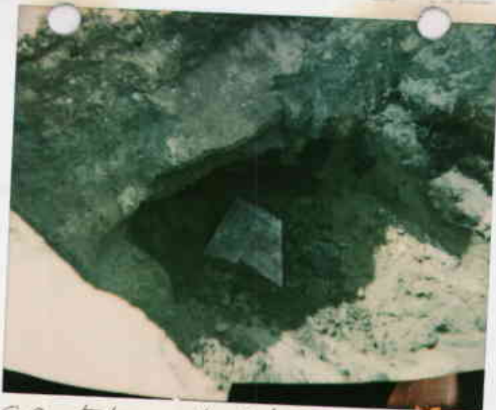
52 taken at 6' bgs 5/3/95 Soil Sample from pit #6 Orotama Sand Dist 1000 gal gas UST 2600 Grant Ave San LO
