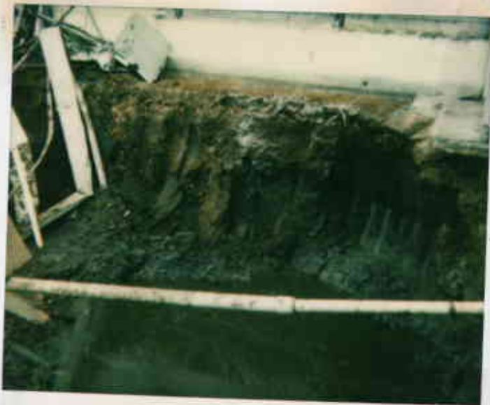
10/20/92 6550 Moraga Ave. sidewall next to fence
