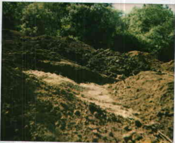
Redwood Regional Park 22215117976-8 6/15/93 Stockpiled soil collected from above tanks. Some contaminated soil accidentally placed in w/ pile. Tuberium 2
