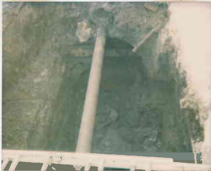
1/10/94 looking north end south - heating fuel tank
