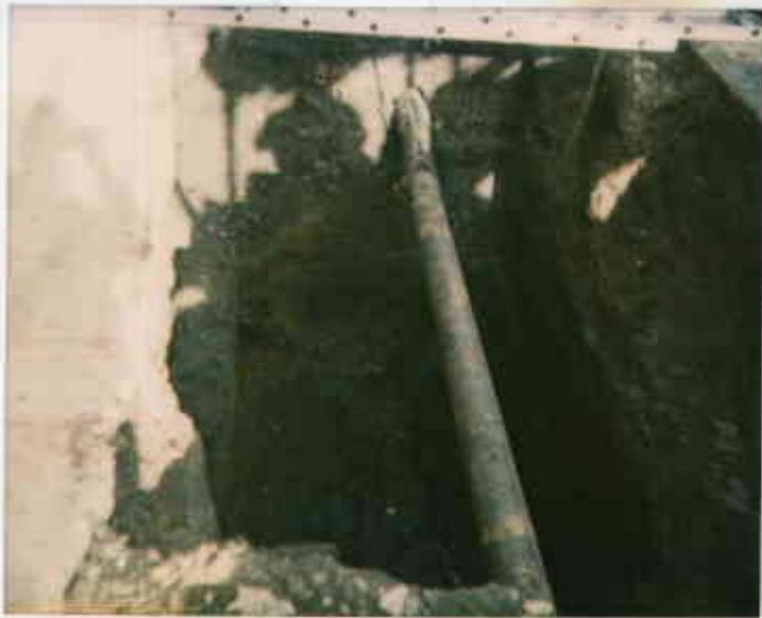
1/12/94 looking from south end north - heating fuel tank
