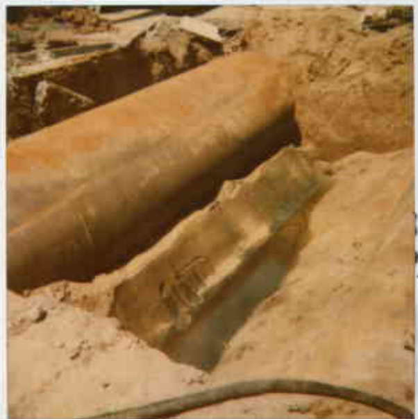
10700 MacArthur - Oak 7/19/94 Middle tank removed - water in pit stained soil Tank 2
