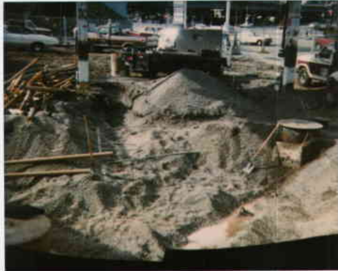
Piping runs Zoo northemont
