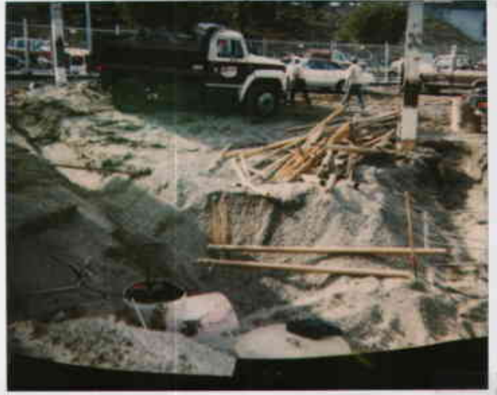
Waste at tank + piping runs
