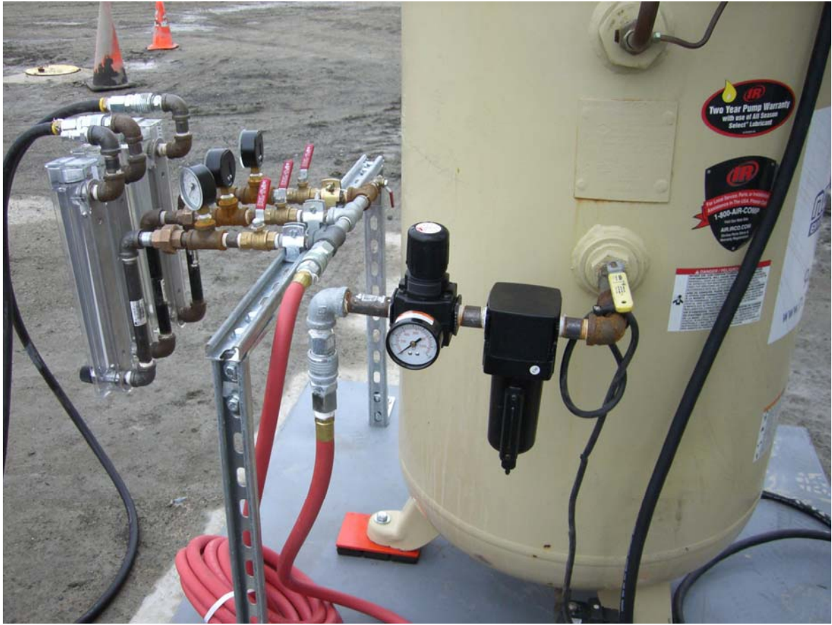
Photograph 2: Air Sparge Pilot Test System Pressure Regulator and Distribution Manifold.
