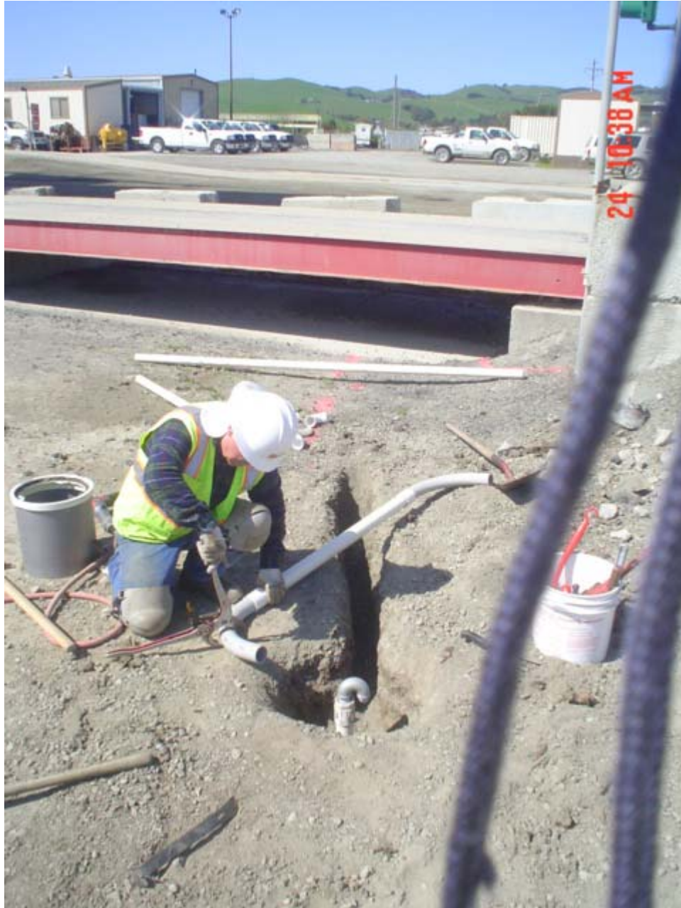
Photograph 1. Injection Well OXY-1D, Compressed Air Hose Conduit, and Trench
