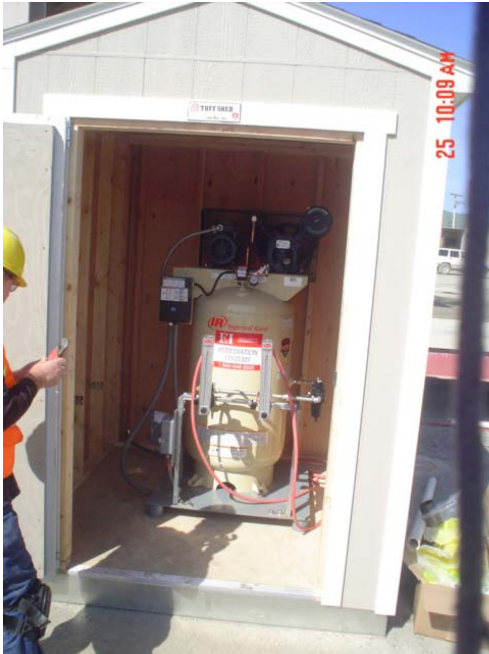
Photograph 2. Air Injection System and Enclosure
