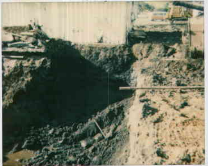
Pit #1, over excavated to Grid 12/18/92, H 2 O coming from under former Pipeline Area
