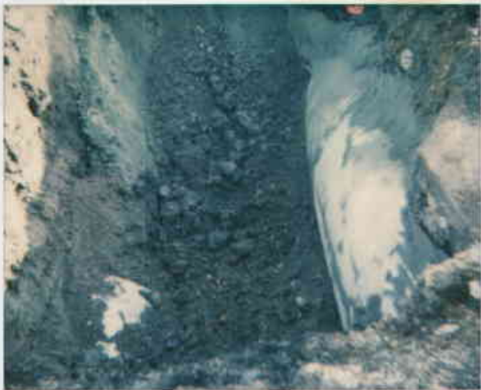
(P) From Hwy Rd looking towards Station. Large storm drain (re) & Sanitary sewer left slightly exposed
