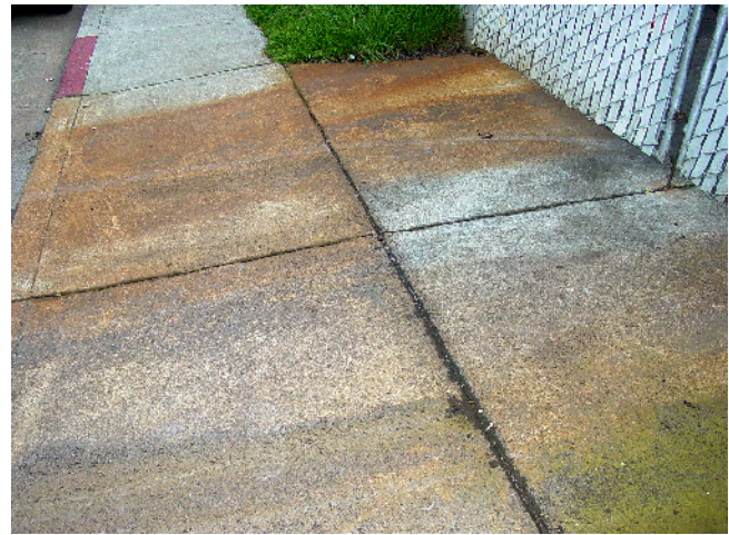
PHOTO 8. Sidewalk stained with rust on Hollis Street in front of the site.
