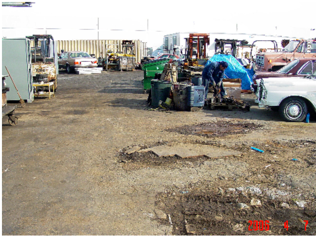
PHOTO 3. Broken Pavement: Some paved areas are deteriorated or missing.
