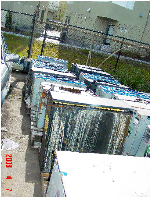
PHOTO 1. Battery Acid: Batteries observed on crates in the southeastern section of the Site. Note that the batteries are uncovered and show signs of corrosion.
