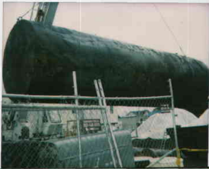
1701 Park St Alameda UST. 4/8/94 One 10,000-gallon UST. No apparent holes or corrosion. 89318221457-2 ASAR 1999 Tutuot Shui
