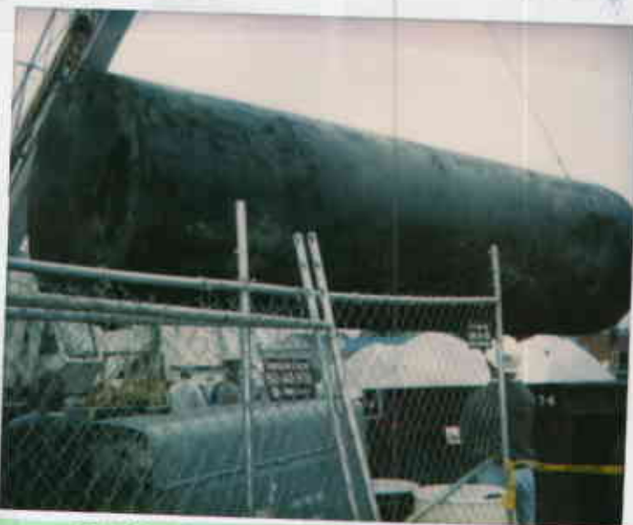
1701 Park St, Alameda 4/8/94 Fourth gas UST, 09318221467-2 removed. No holes 1992 N ← S 0000 Juliet Shinn
