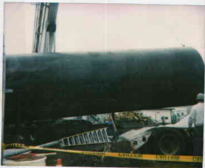
1701 Park St., Alameda 4/8/84 Incl gas UST removed 09318221467-2 NE 35 ✓ No apparent holes JULIET SLUIJ 00000
