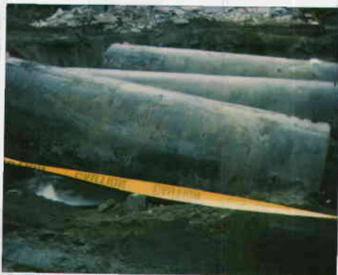
1701 Park St, Alameda 4/8/94 Four 10,000-gallon USTs removed. One gas and 3 One diesel and three gas. Water in pit Tutuot Shui
