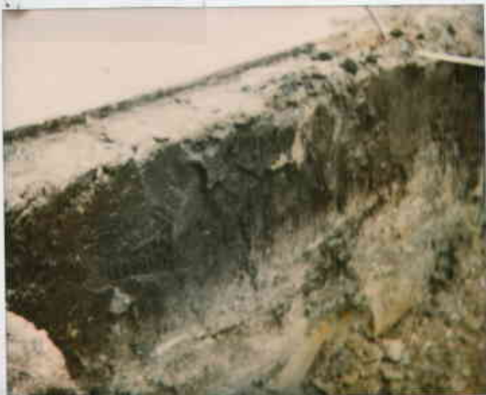
10/25/96 ST 103314 04618111090-24 1348 7856 On site - hot area COPIES & ENLARGEMENTS CALL 800-421-1030 + removal of dispenser cabinet
