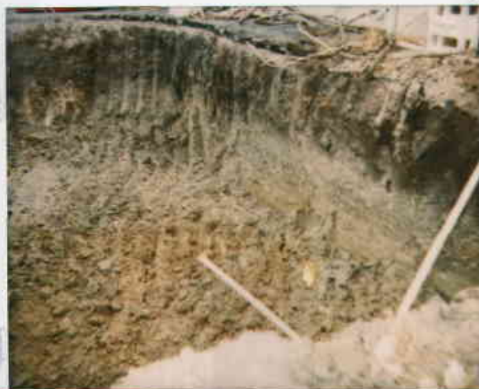
10/25/96 ST 103314 04618111090-24 1348 7856 Over site - hot area COPIES & ENLARGEMENTS CALL 800-421-1030 removal of old dispenser cabinet
