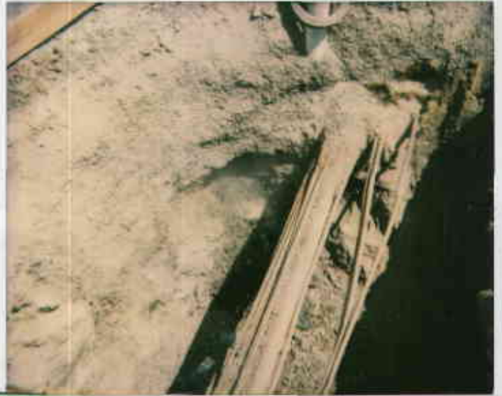
7/20/93 Photo taken by Ron Owcasz at shell station @ 2120 Montana Ave. in Oak for piping of UGT work where soil contamination was found at pit overexcavation. ©
