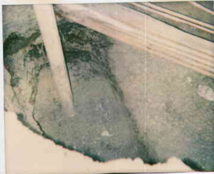
7/20/93-Photo taken by Ron Owcasz at Bangal shell, 2120 Montana Ave. Oak. Shown is soil cont. at side wall of pit overexcavation for UGT pipe work. ©
