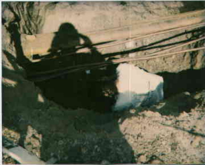
7/19/93-Photo taken by Ron Oweasz at Banzal Shell, 2120 Montana Ave, Oak. Shown is Allison Watts taking soil samples at pit overexcavation. ©
