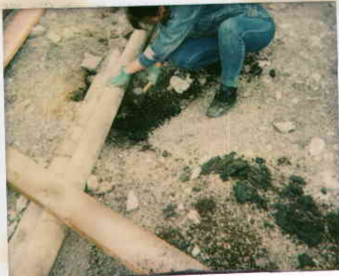
7/6/93-Photo taken by Ron Owcasz at Banzal shell, 2120 Montana Ave. Oak. Shown is Allison Watts taking soil sample under middle of old piping where some soil cont. was observed. 12215117976-B
