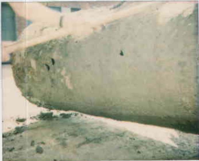
Gasoline tank 7/28/94 Obvious holes 2417 Broadway
