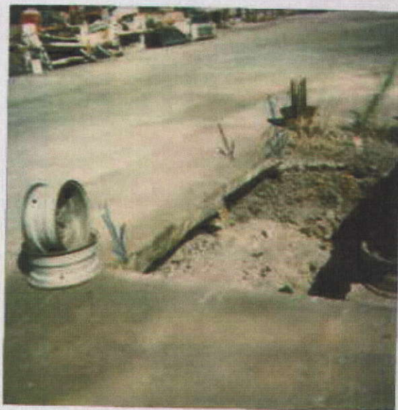
3744 Depot Rd. Hayward 8/29/95 Location of soil borings collected from waste oil tank pit
