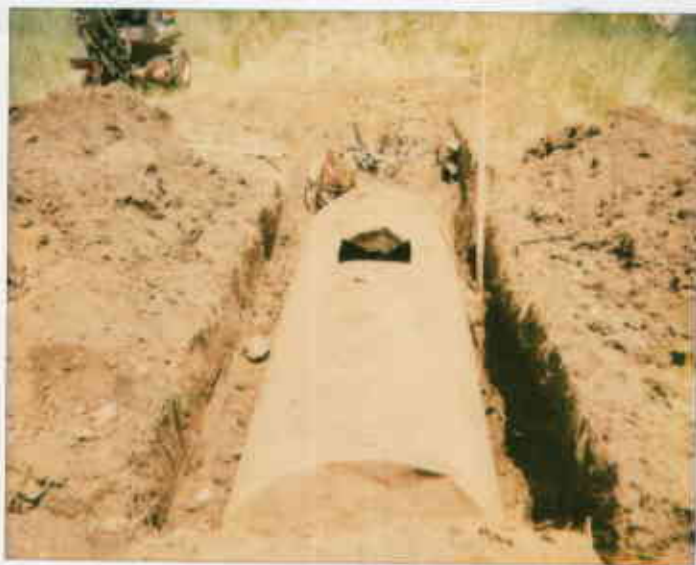
6159 Kaew, 1000 gal fuel oil tank Tree stump preventing tank removal
