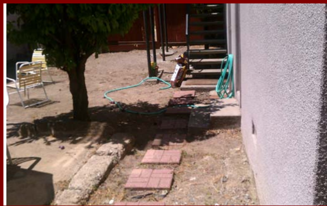
Back of Apartment Building at 5320 Coronado (Note vent and unimproved ground surface)
