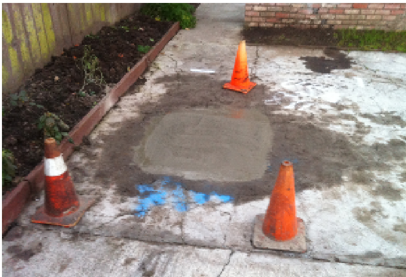
5 January 2012. View of well MW7 after decommissioning/abandonment and subsequent pavement repair. The well casing was cut off \pm 1 -foot below top of pavement, the wellhead vault was removed, the concrete pavement was sawcut, and concrete was placed.
