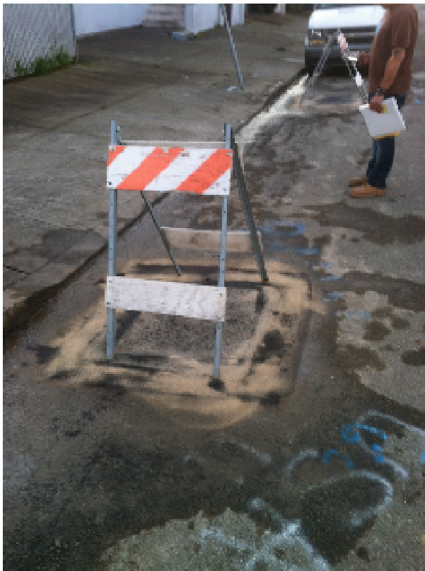
5 January 2012. View of wells MW5 and MW6 after decommissioning/ abandonment and subsequent pavement repair.
