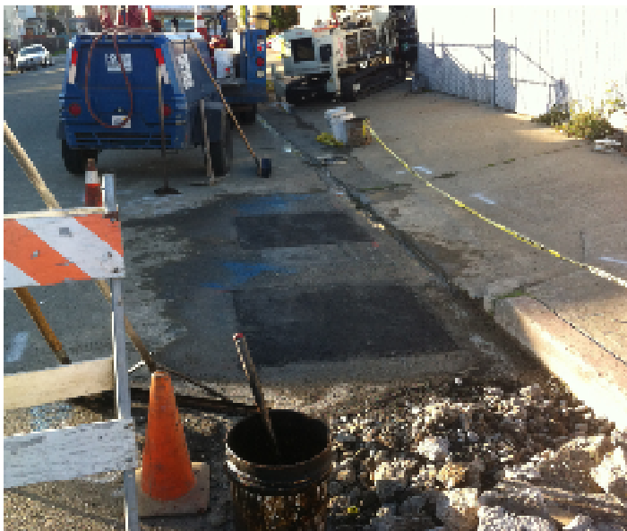
5 January 2012. View of wells MW2 and MW4 after decommissioning/ abandonment and subsequent pavement repair.
