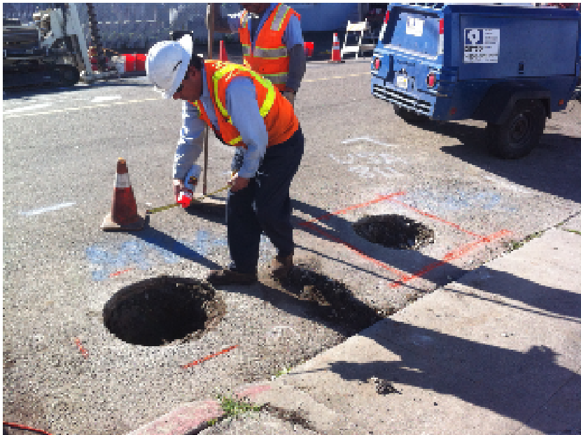
5 January 2012. View of wells MW2 and MW4 after grouting and overdrilling to a depth of 5 feet.
