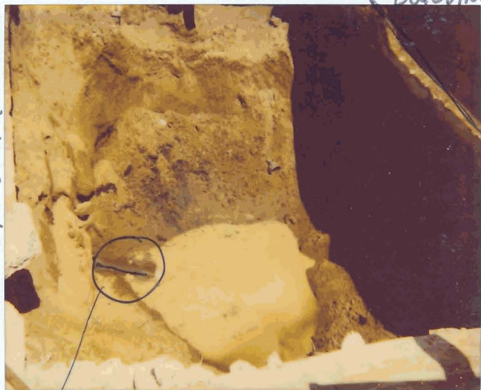
2124 LIVINGSTON OAKLAND BROKEN SEWER PIPE 4-16-98 PW
