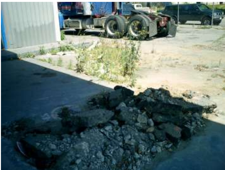
Photograph No. 3 - view westward of canopy area showing trench from dispenser and product piping removal. Former USTs located under location of power unit parked in background.
