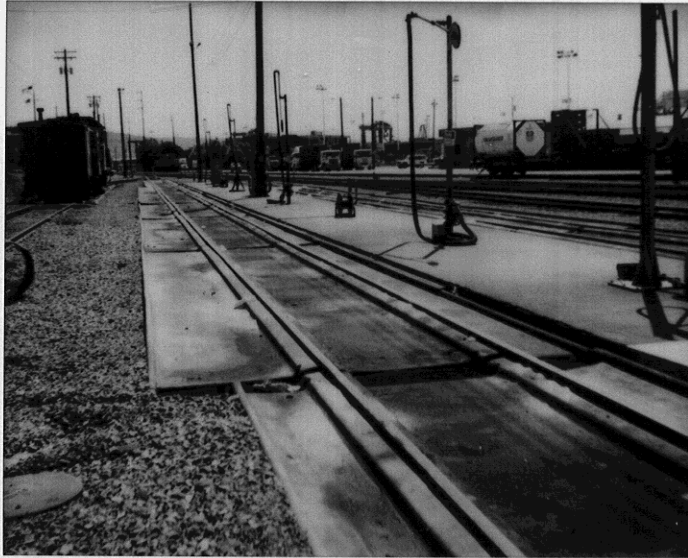
5-13-93 UPRR JK 1717 Middle Harbor Rd. diesel filling area
