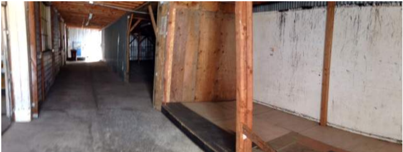
Photo 18: Subject Site (Facing Northeast) 3820 Penniman Avenue Exterior Associated Paved Area - Storage Shed
