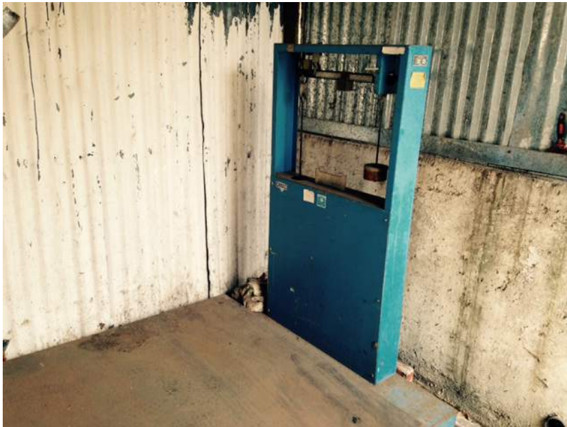
Photo 22: Subject Site (Facing North) 3820 Penniman Avenue Exterior Associated Paved Area and Storage Shed - Scale
