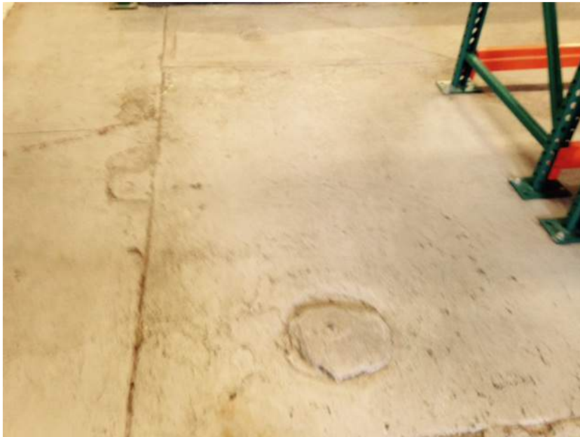
Photo 24: Subject Site (Facing Southeast) 3820 Penniman Avenue Interior Storage Warehouse - Former Underground Lift
