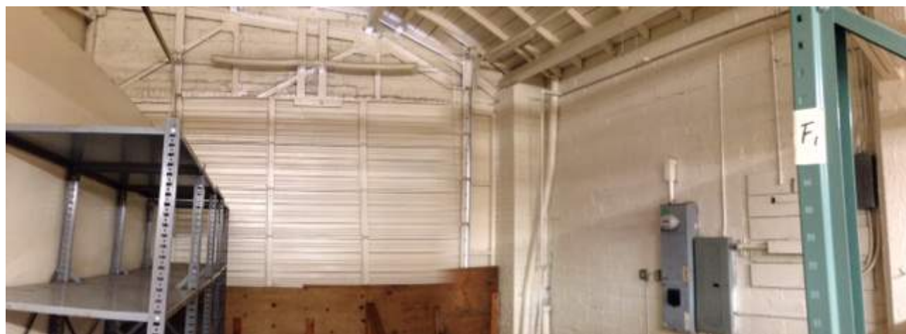
Photo 10: Subject Site (Facing Southwest) 3820 Penniman Avenue Interior Storage Warehouse - Roll Up Door
