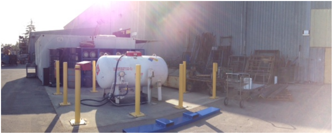
Photo 23: Subject Site (Facing Southeast) Propane Above Ground Storage Tank
