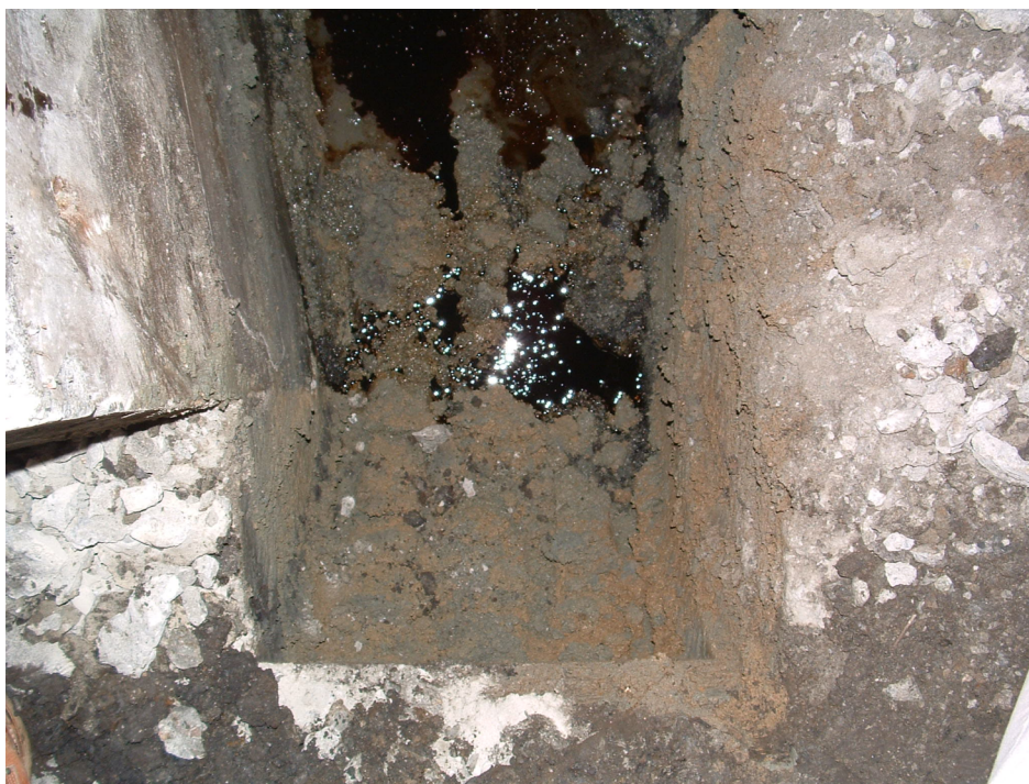
Fig. 1. Photograph of the hydraulic fluid released from the gravel zone around the ring roller foundation.
