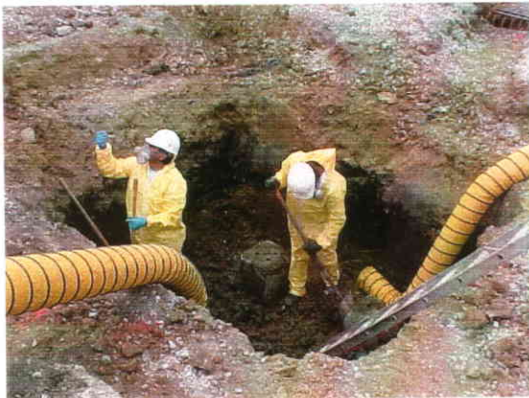
Figure A5. Using blowers to supply fresh air into the contaminated pile caps
