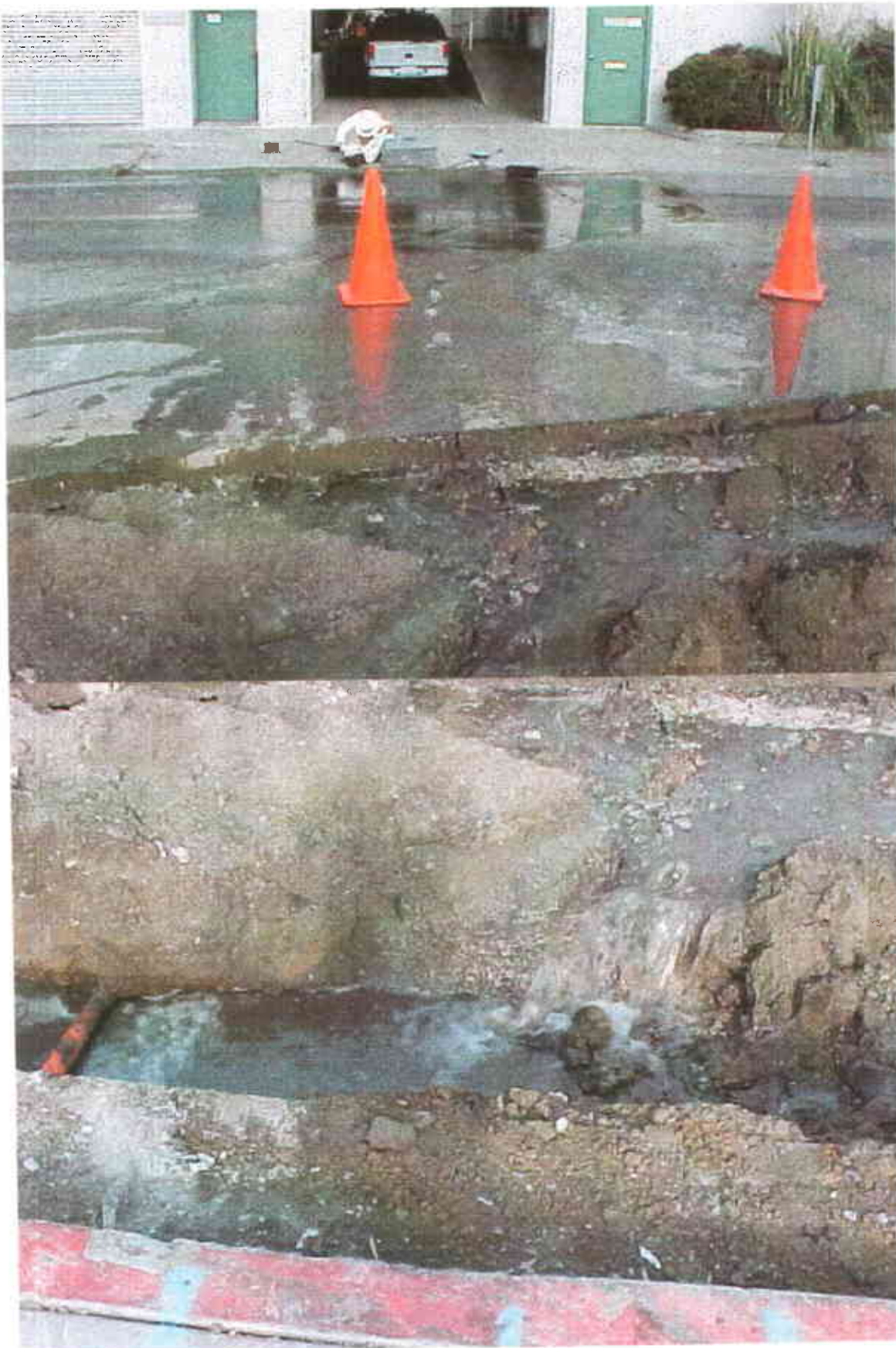
Stormwater Entering the Trenches
