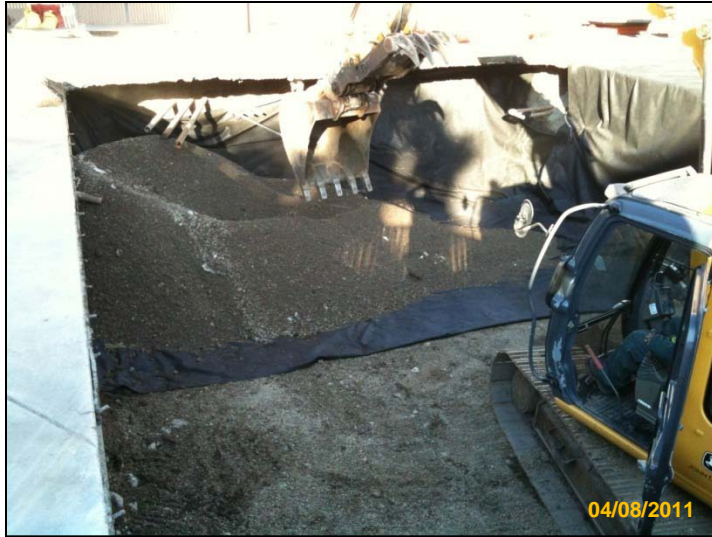
PHOTO 45: Adding pea gravel on top of fabric on west end of excavation.
