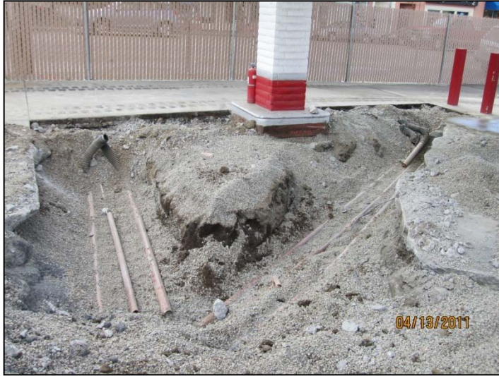
PHOTO 53: Product lines (x2) and return line to Dispenser #1 (Pumps 1 and 2) to the left, and Dispenser #2 (Pumps 3 and 4) to the right. Piping set at 2 feet bgs, with pea gravel extending to 3 feet bgs.
