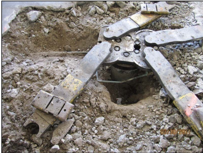
PHOTO 9: Air line exposed to east hoist.
