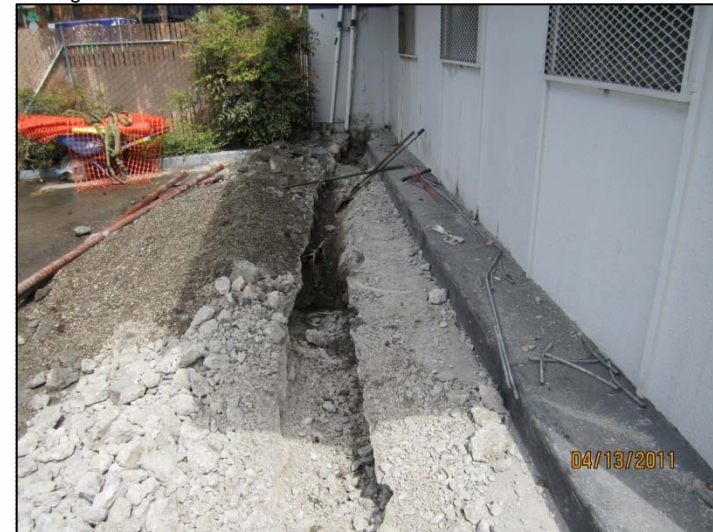
PHOTO 56: Removing both vent lines along west side of station building. No indication of a fuel release.
