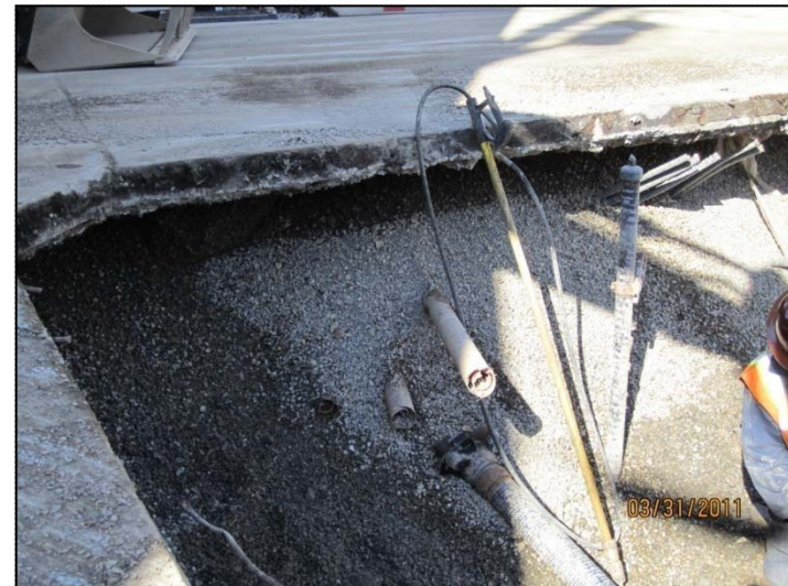
PHOTO 20: Product piping, return piping, and conduits heading to two dispensers along College Avenue (Pumps 5 through 8).
