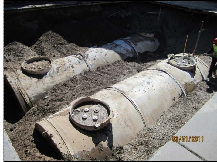
PHOTO 26: Overview of exposed fiberglass-coated steel USTs looking south. Near tank is 15K super unleaded. Top of tanks is roughly 6 feet below grade. Four straps on each tank.
