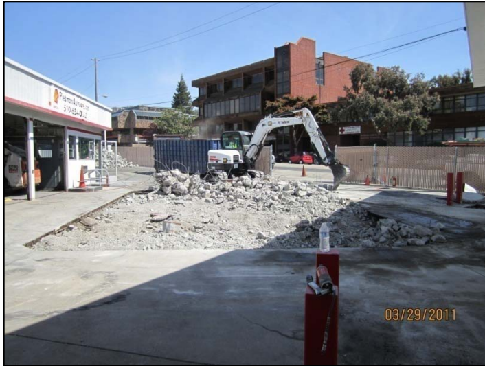
PHOTO 1: Breaking and removing concrete slab from atop UST pit, looking east-northeast. Area measures 25' wide by 35' long.
