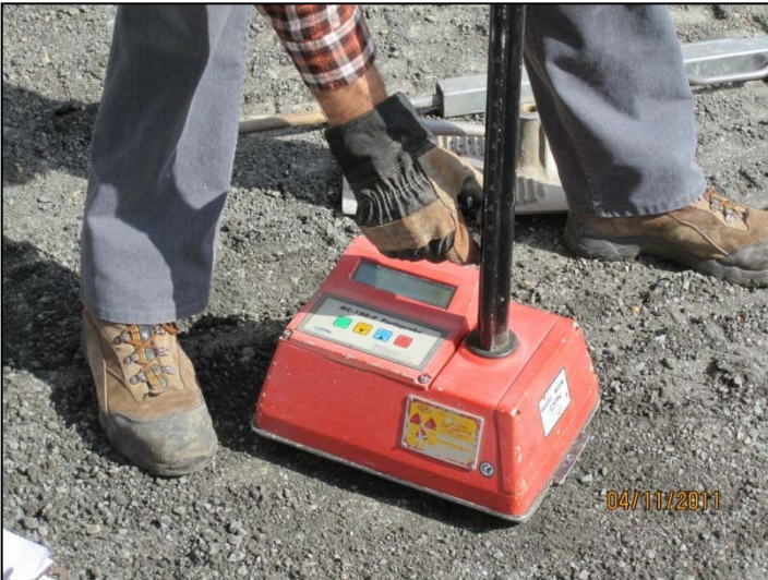
PHOTO 51: Compaction testing during backfill. 90% relative compaction achieved below 4 feet. 95% relative compaction achieved 0-4 feet (in one foot lifts).
