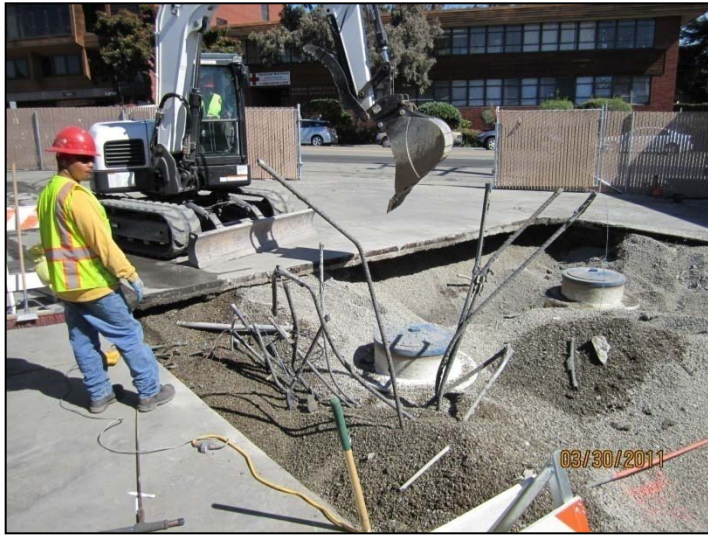
PHOTO 13: Electrical conduits exposed in northeast corner of UST pit, just above the 15K super unleaded UST.
