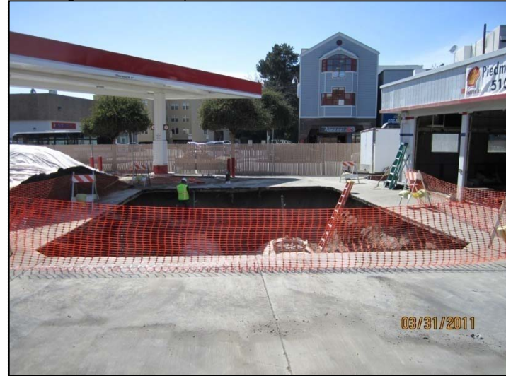
PHOTO 28: Overview of 25' x 35' UST pit being cordoned off with orange construction fencing.
