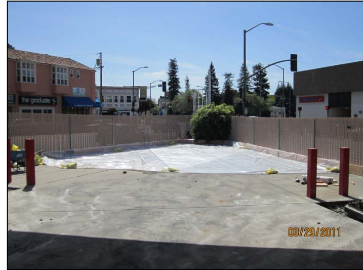
PHOTO 2: Staging area in southern tip of Site, for temporary storage of pea gravel from UST excavation.
