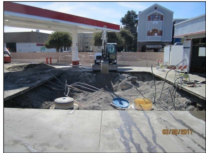
PHOTO 14: Overview of partially excavated UST pit, looking west-southwest. 15K super unleaded UST is on the right; 20K regular unleaded UST is on the left.
