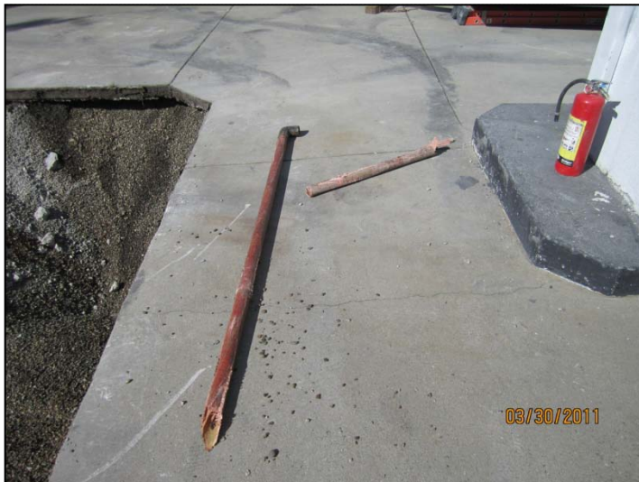
PHOTO 11: One of two single-wall fiberglass UST vent lines removed in northwest corner of UST pit.
