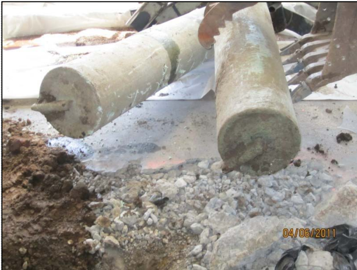
PHOTO 43: Base of hoists – east hoist on the left, after draining. West hoist on the right, before draining.
