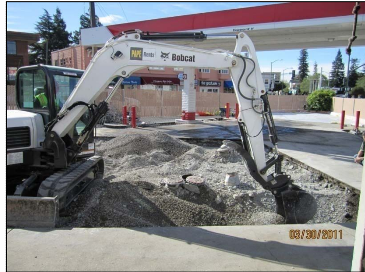
PHOTO 10: Beginning excavation of pea gravel in northwest corner of the UST pit.
