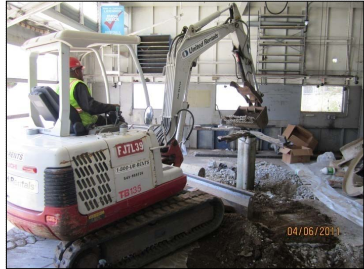
PHOTO 42: Pulling west hoist. Both hoists were fiberglass coated steel units, with no indication of leaks.
