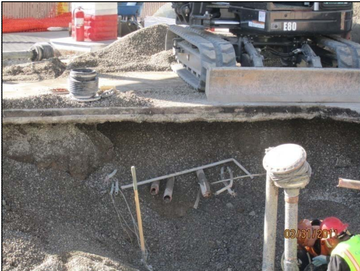
PHOTO 19: Product piping , return piping, and conduits heading to two dispensers along Claremont Avenue (pumps 1 through 4). Product and return piping is dual-wall fiberglass.
