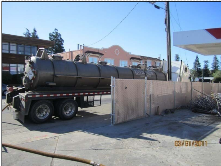
PHOTO 15: EnviroServ vacuum tanker truck on site for steam cleaning of both USTs (triple rinse).
