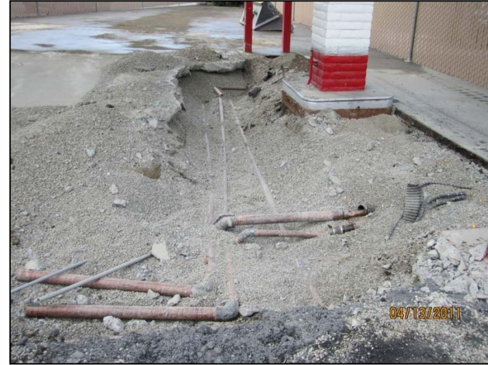
PHOTO 54: Product lines (x2) and return line to Dispenser #3 (Pumps 5 and 6) in background and Dispenser #4 (Pumps 7 and 8) in foreground.
