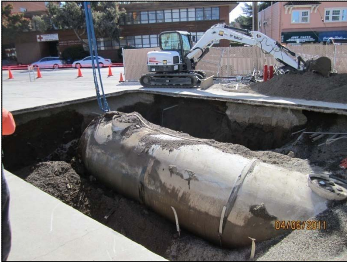
PHOTO 37: Freeing east end of 20K UST before pick. 200 lbs of dry ice was added before pick, preceded by 60 lbs of compressed CO2 gas.
