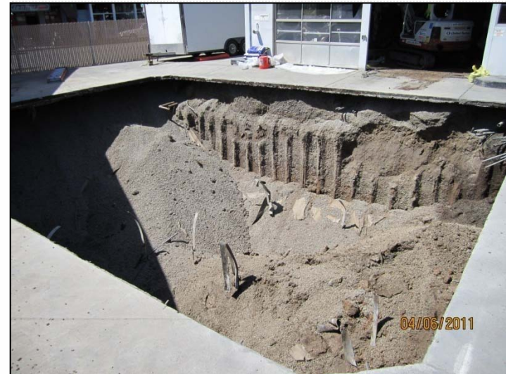
PHOTO 44: UST pit after tanks removed. Note pea gravel which has sloughed in from west end of excavation.
