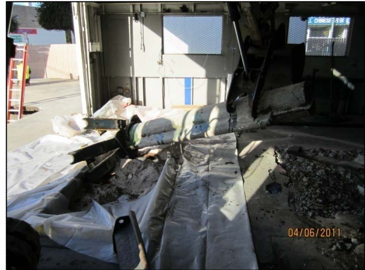
PHOTO 30: Draining hydraulic fluid from east hoist. Drainage basin was created in former dynamometer pit, using plastic sheeting and granular absorbent.
