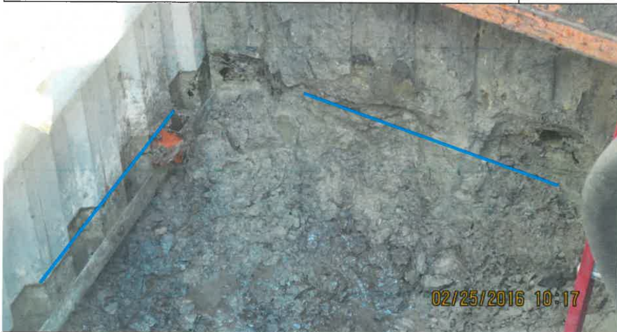
DESCRIPTION: HOLE WHERE NORTH WALL SOIL SAMPLE WAS TAKEN – JUST ABOVE GROUNDWATER LINE.
