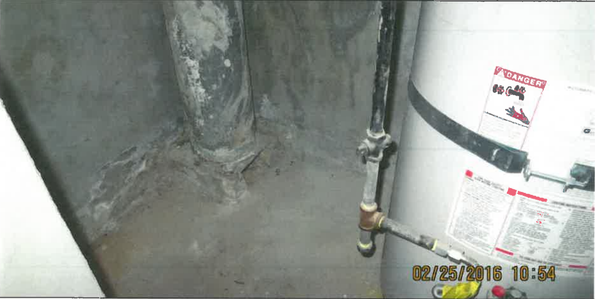
DESCRIPTION: SENIOR CENTER BUILDING BASEMENT VIEW AROUND WATER HEATER (EAST SIDE OF BUILDING) NO PIPING Photo # 18 of 25
