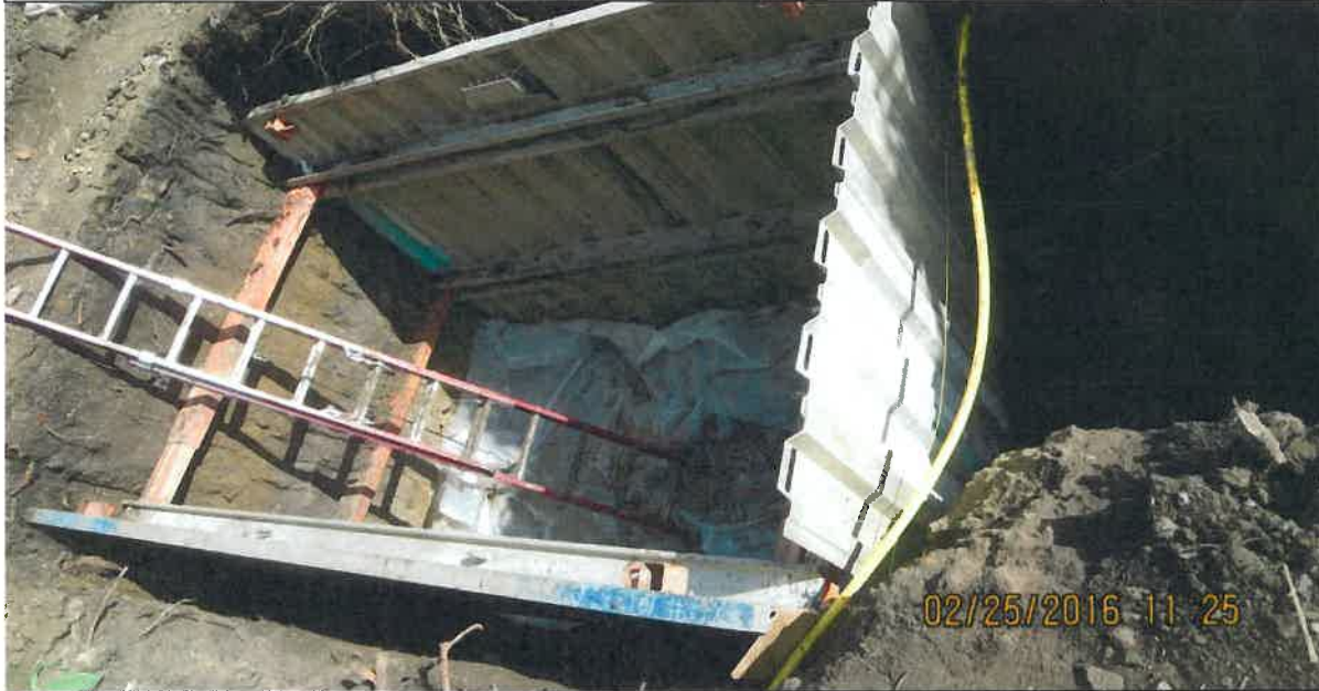
DESCRIPTION: LINER PLACED OVER UST CLOSURE PRIOR TO BACKFILL WITH PEA GRAVEL Photo # 24 of 25
