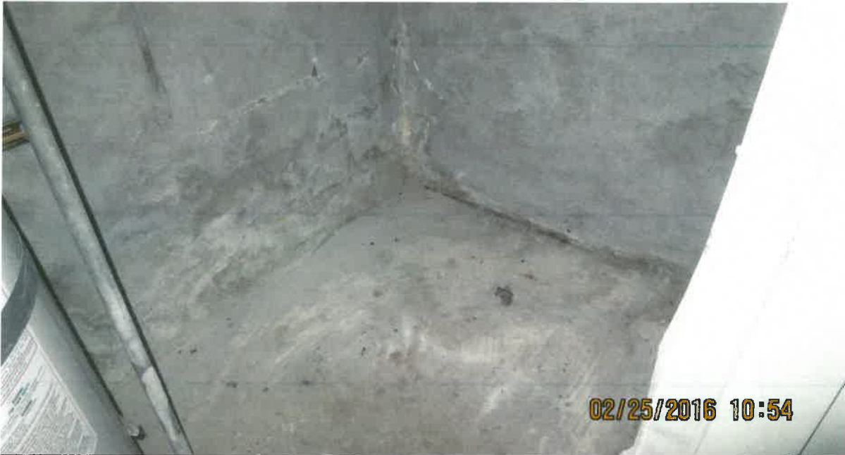
DESCRIPTION: SENIOR CENTER BUILDING BASEMENT VIEW AROUND WATER HEATER. (EAST SIDE OF BUILDING) NO PIPING Photo # 17 of 25
