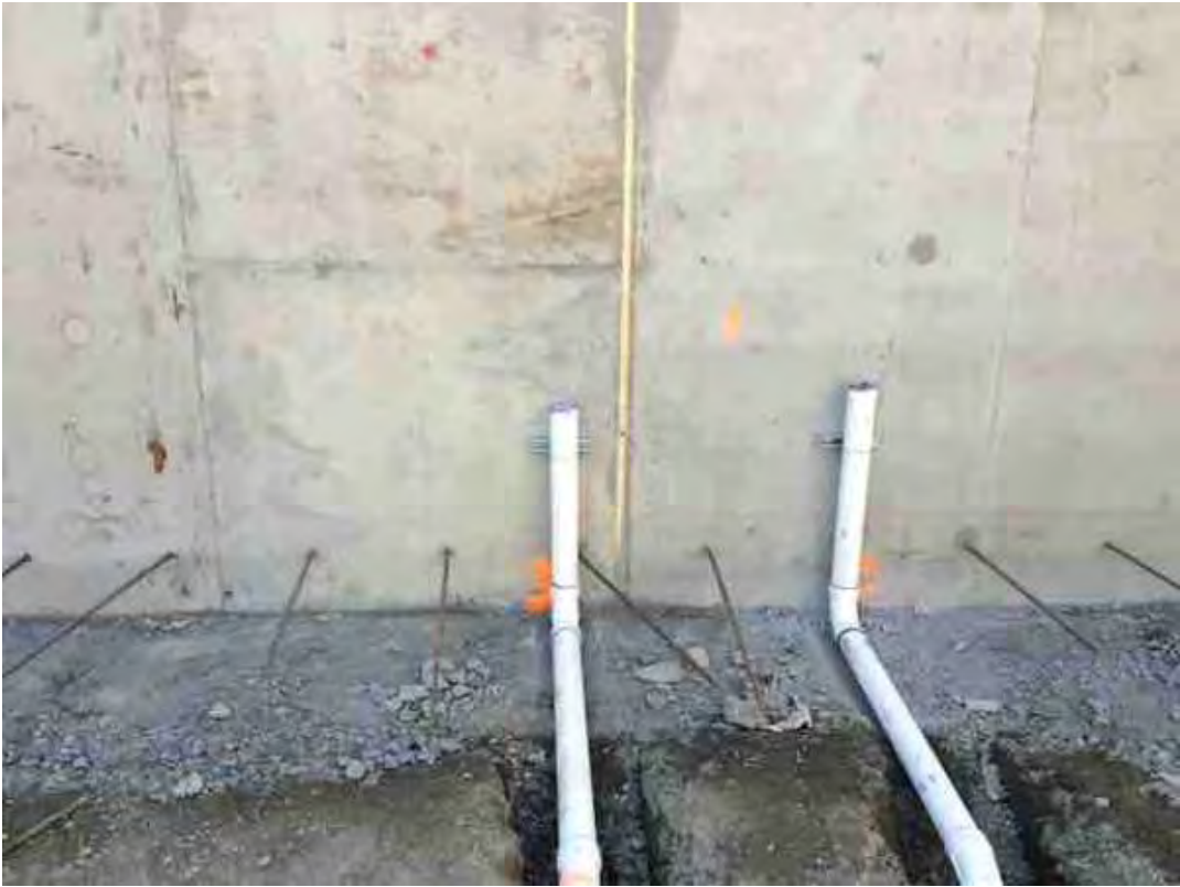
They have wood in the walls the need grouting.
