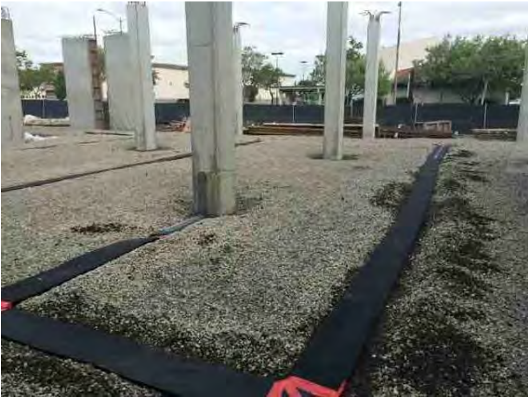
Installed our vent system
