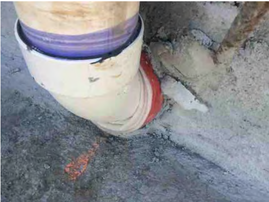
Plumbing pipes with the sleeve need to be grouted
