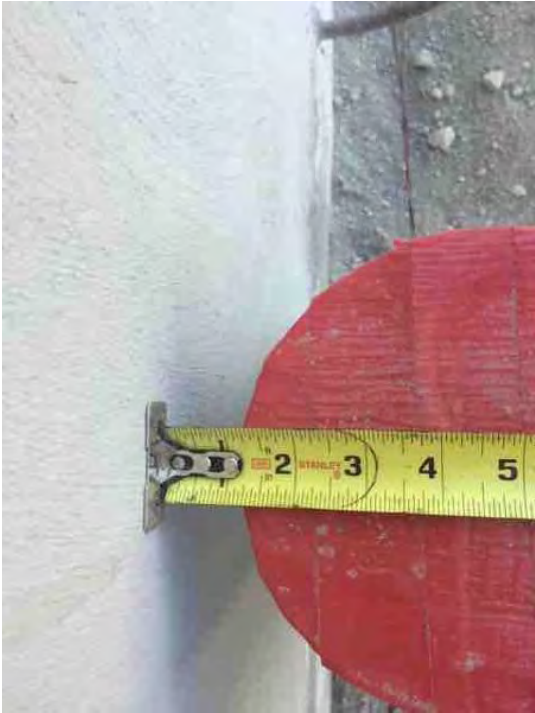
Plumbing pipe and it's a inch away from the wall
