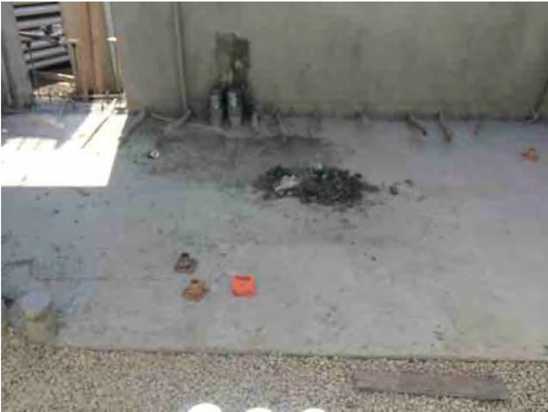
Dirt needs to be removed
