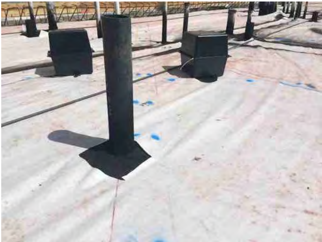
On pad pad D-2 concrete foreman was off with his measurements so Dan what's two 90s to try to correct it
