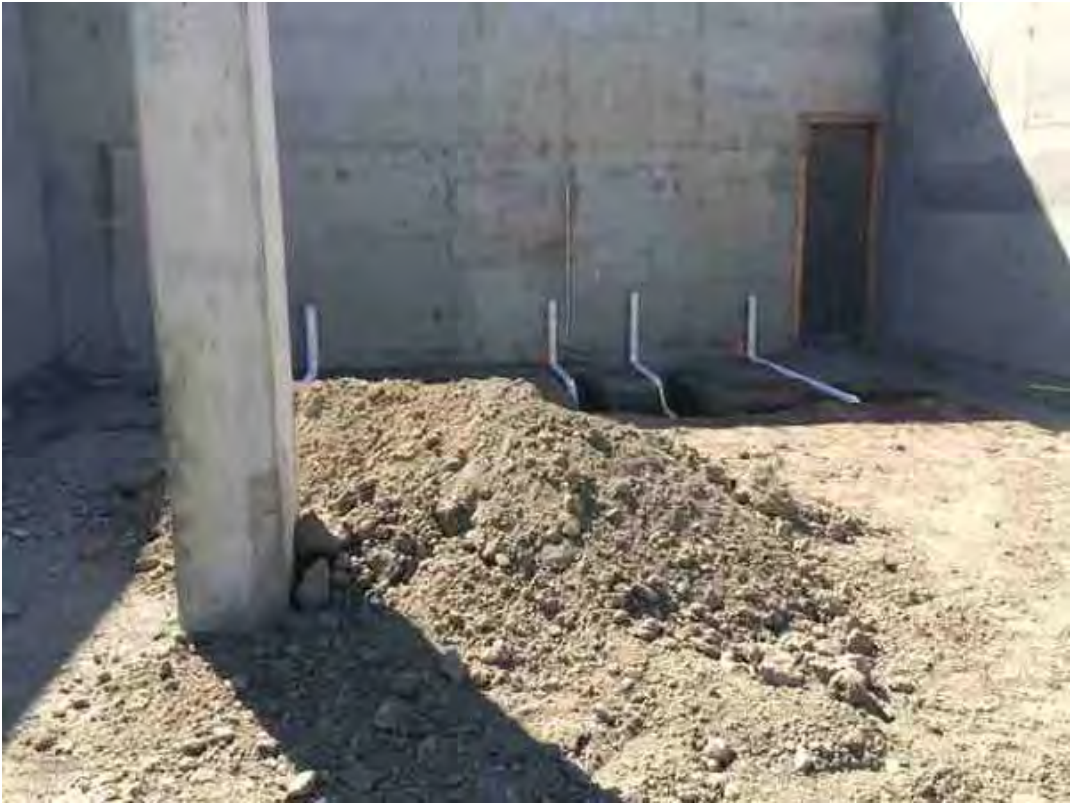
Pad F isn't ready. They need to backfill the pipes and grade it.
