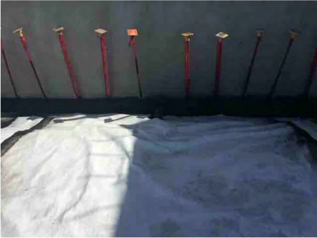
Patched in section where they cored the wall
