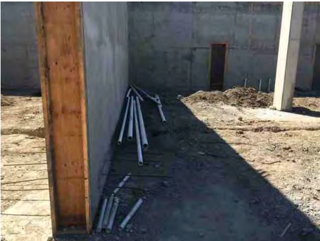
Areas need cleaned out and graded
