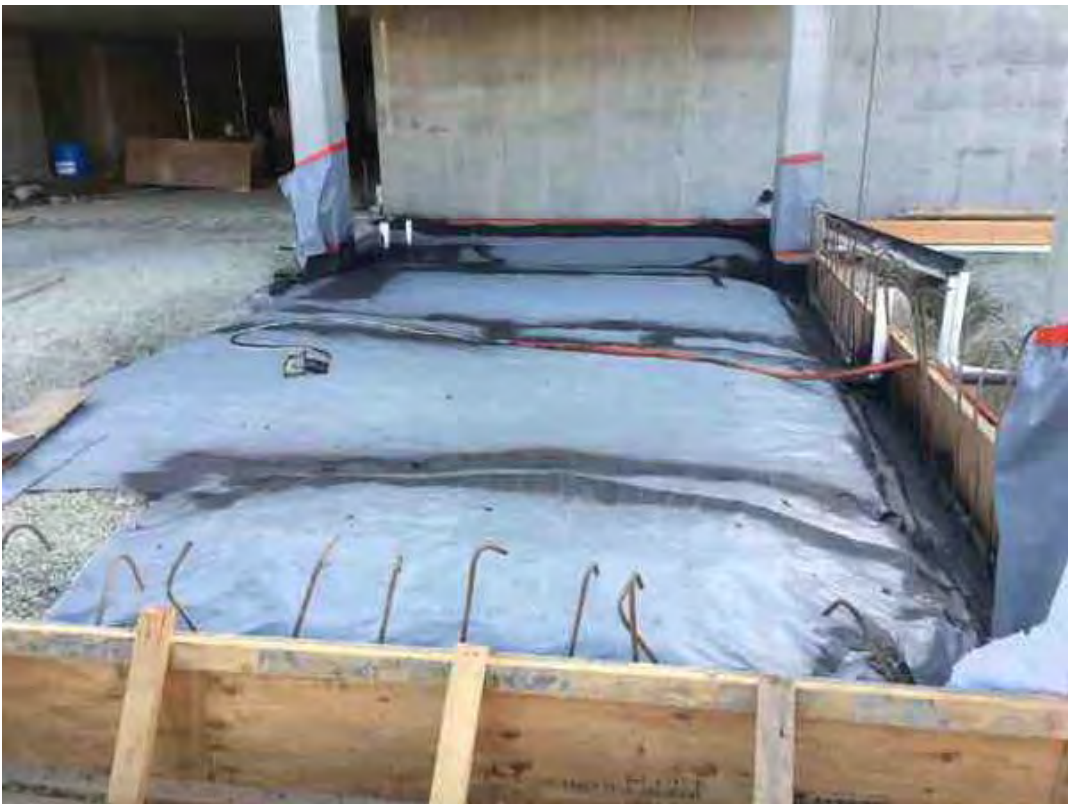
Installed base in mail room
