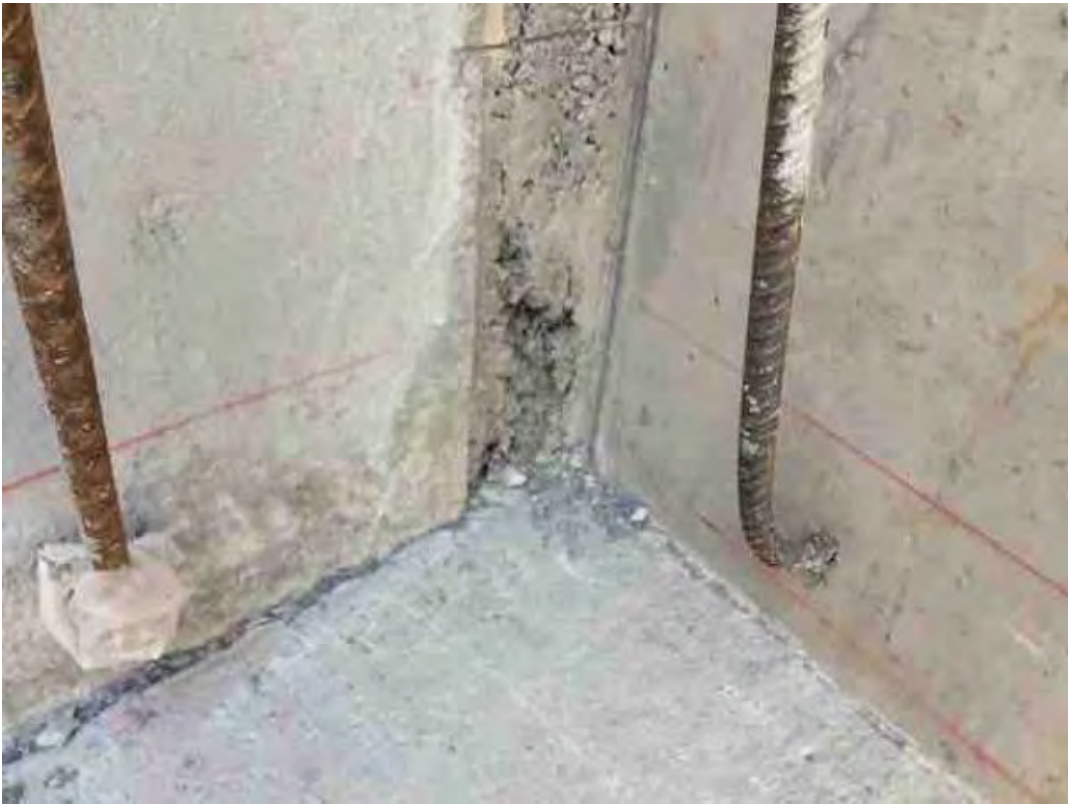
Corners need grout
