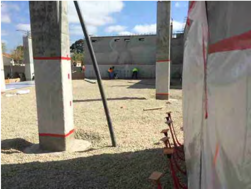
Concrete guys remove the rock in the footings for our 6 inch Tie in
