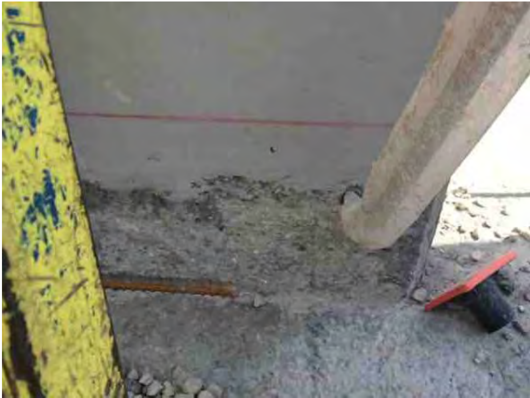
Wall needs grout
