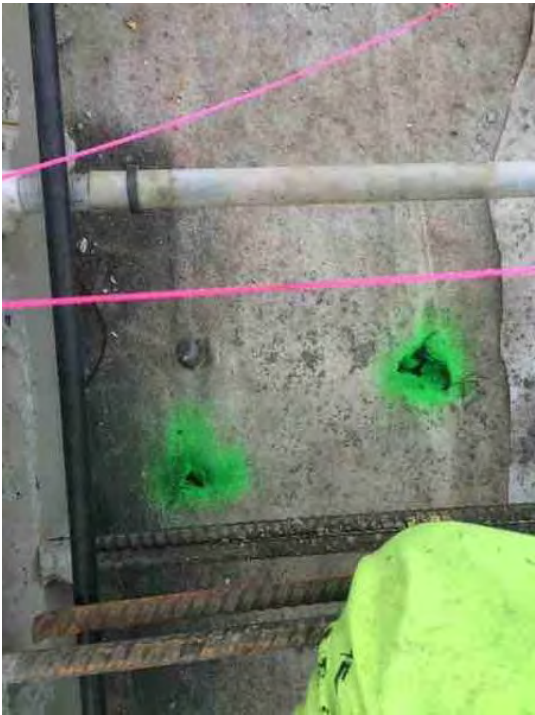
Lots of steaks are pulled out the pad and there's holes
