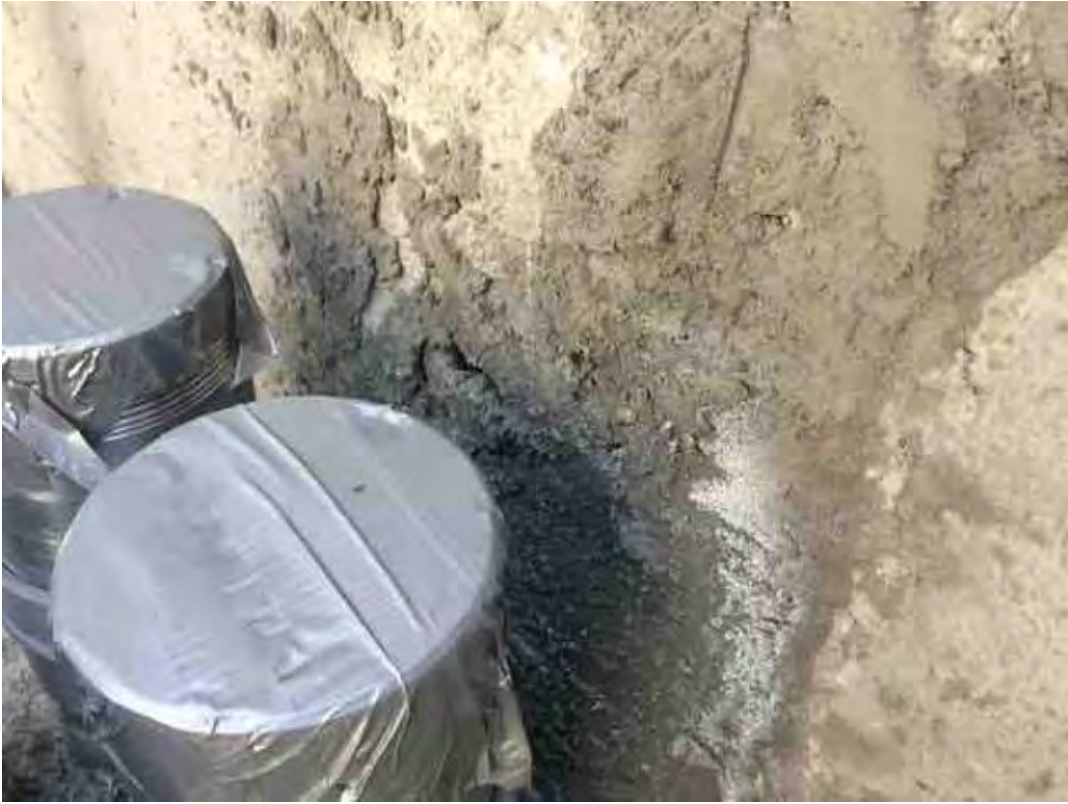
Pipes still need grout
