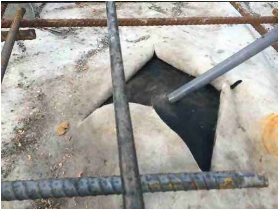
The rebar guys or angling the steaks and the pad is pulling up and it's loose
