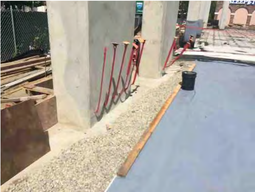
Stopped 3' from the footing and started spraying out the pad with mill incase it rains
