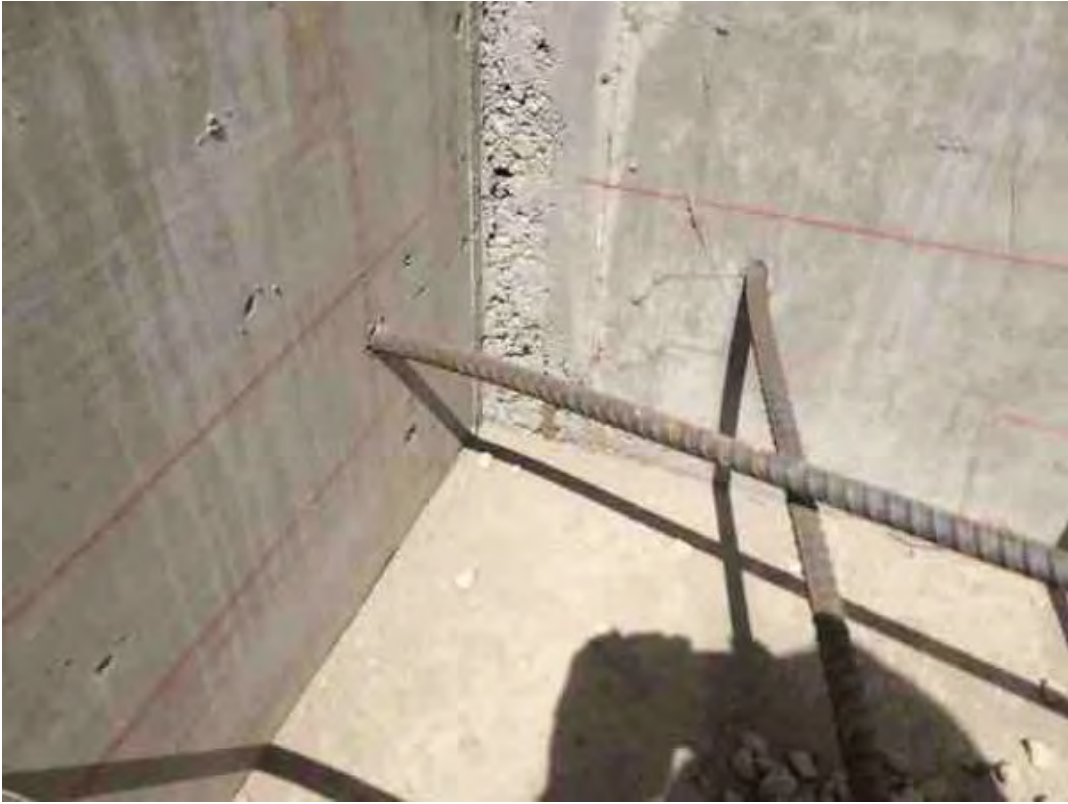
Corner needs grout
