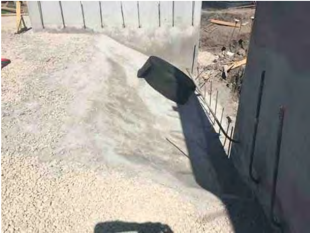
Top of the concrete is a little rough. Dan said they're going to put gravel on top of it it'll go away
