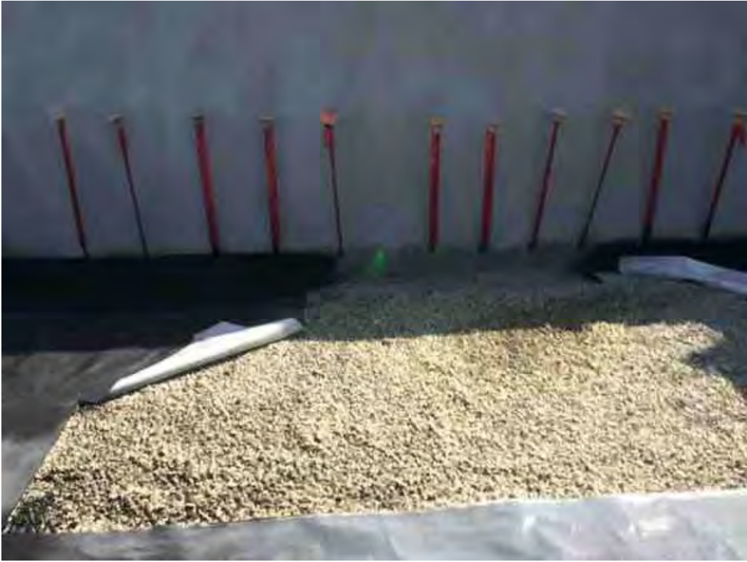
Left out section because wall needs cored
