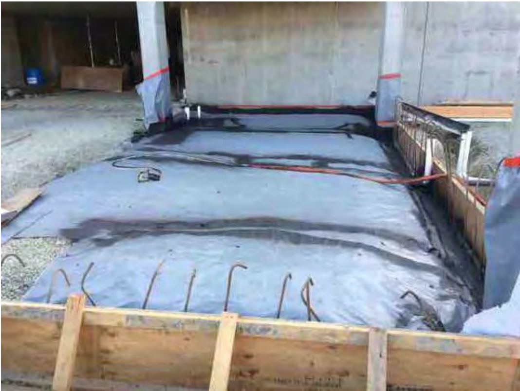
Installed base in mail room
