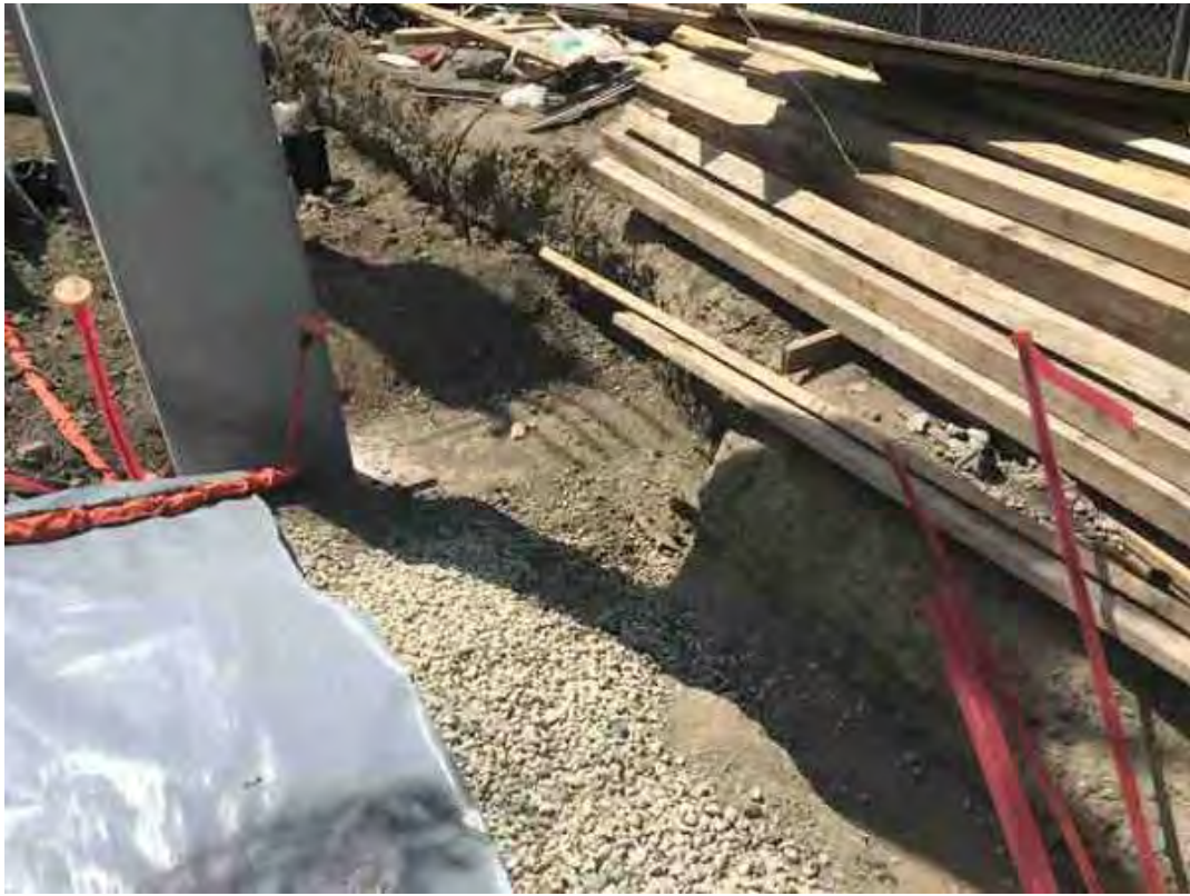
All I have is 3' of material tie end
