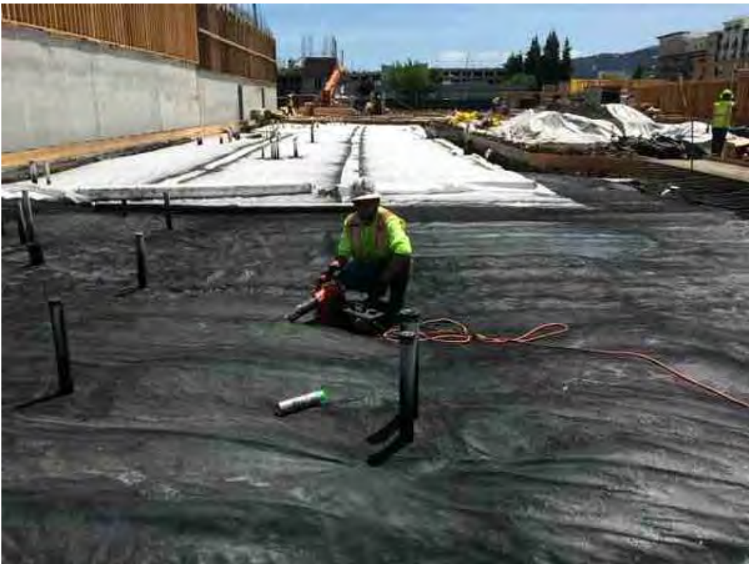
Pre smoke test
