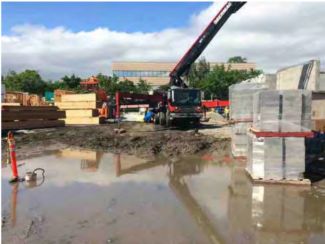
And there's a concrete pump truck in our way so we can't leave
