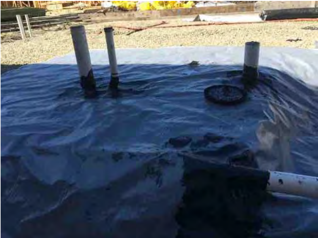
Detailed pipe penetrations
