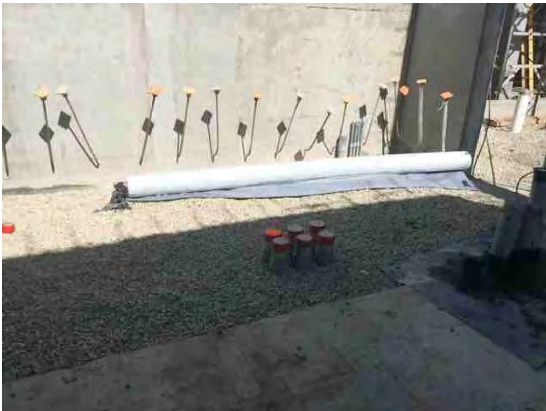
Electric room is what's left
