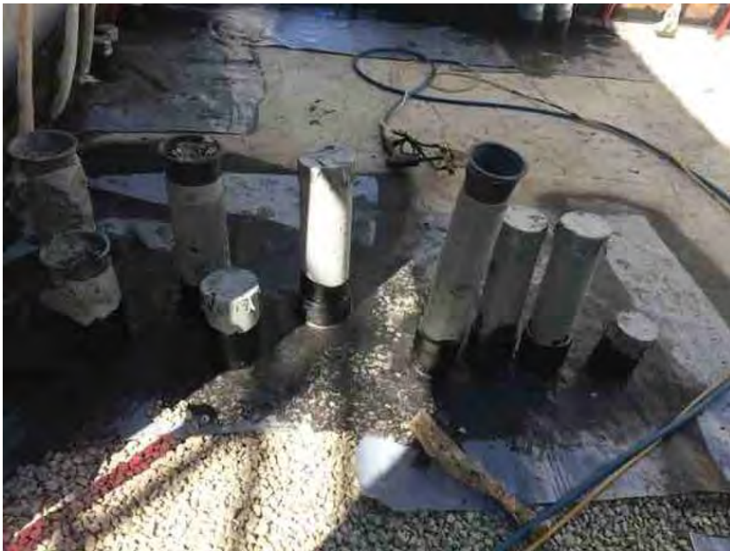
Finished installing all the penetrations and installed our vapor pad and smoke tested it with Dave Devine
