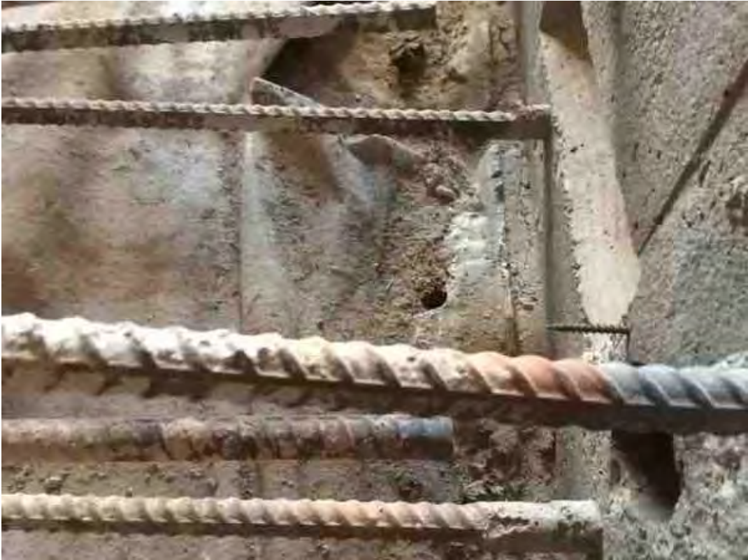
Need to patch vapor steak holes
