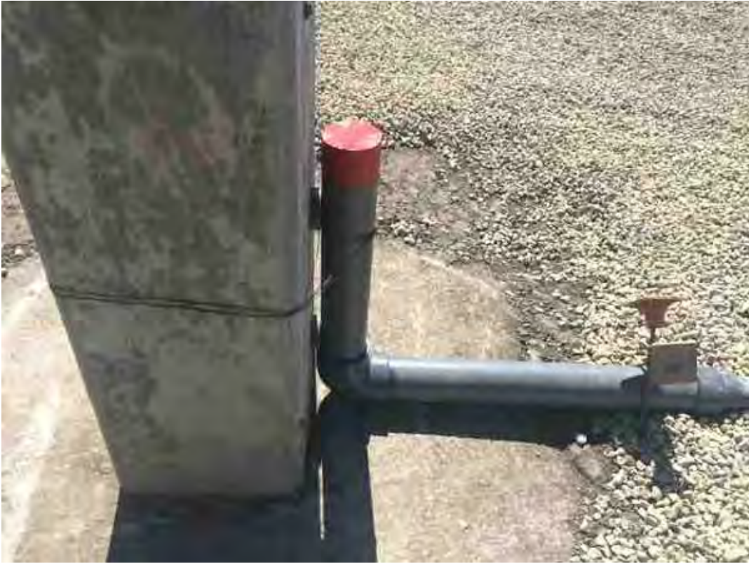
Are riser pipe they want and it's away from the wall
