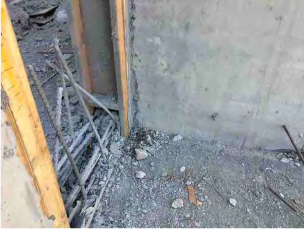
Corners of the walls need grout
