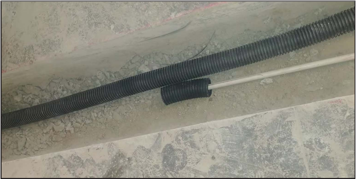
Photo 3 - SSV Piping and Sub-slab Probe with Protective Outer Casing
