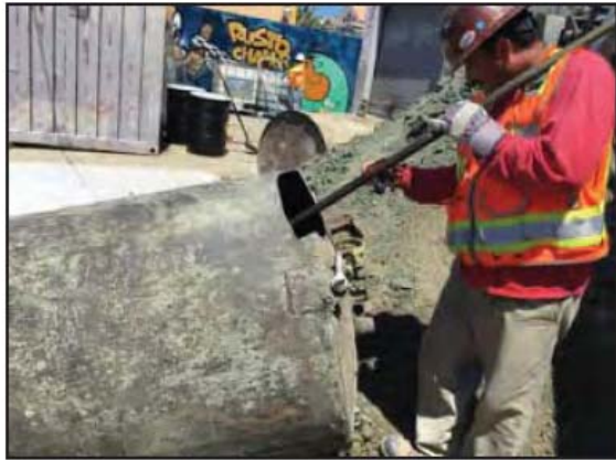
Photograph 13: A hole was cut into the fourth UST and was then triple rinsed by Western Abatement personnel.
