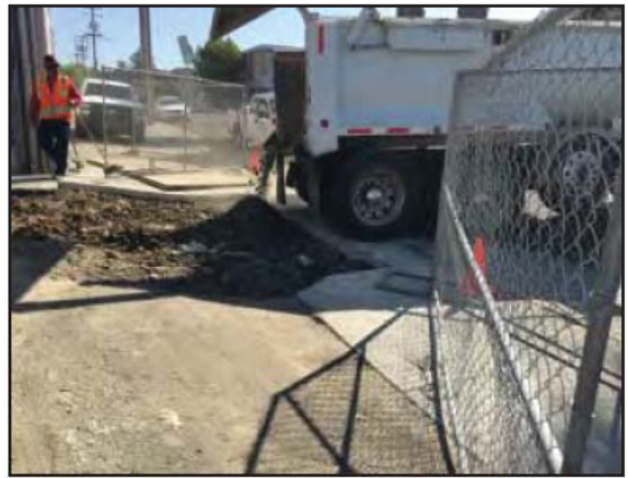
Photograph 16: Clean imported fill was also added to the UST pit to make up for the volume of the USTs.
