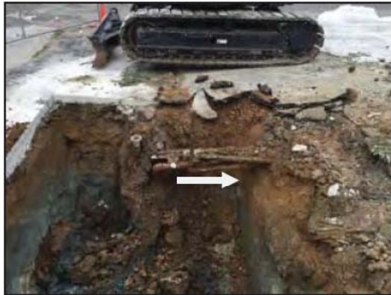
Photograph 9: Multiple pipes were found running northwest (arrow) into the subject property and southwest towards the fifth UST.
