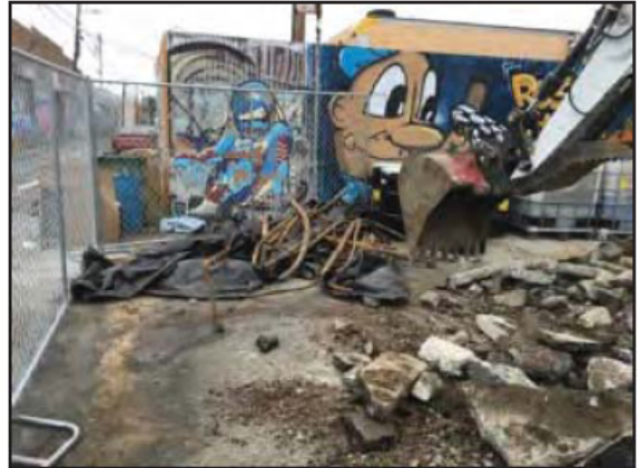
Photograph 28: Approximately 200 ft of piping was removed and stored on a plastic liner before disposal.
