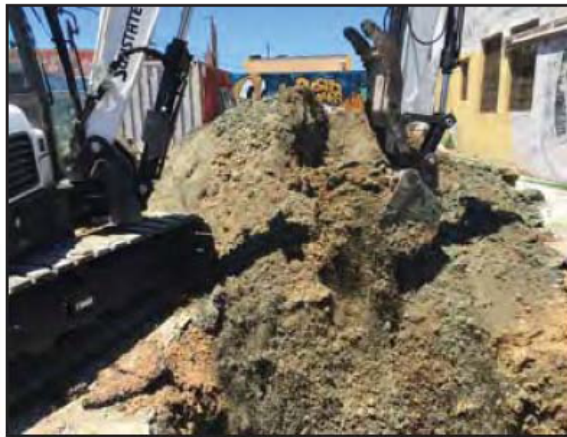
Photograph 15: The third and fourth UST pit was temporarily backfilled using the stockpile soil, which will later be removed during over-excavation.
