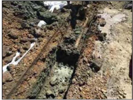
Photograph 26: Trenches were excavated along the piping system for sampling and removal of the piping. Note the shallow olive green soil staining.
