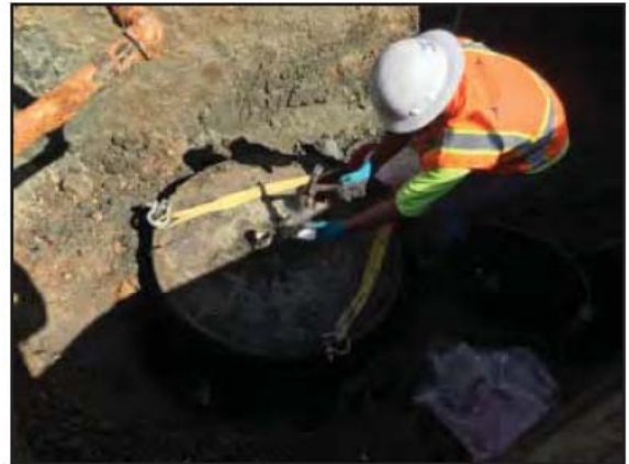
Photograph 10: Dry ice was added to the fourth UST to lower the oxygen level and Lower Explosive Levels (LELs).
