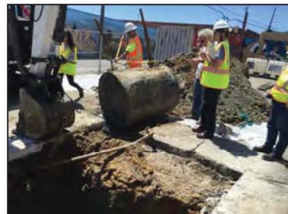
Photograph 4: Residual soil was scraped off of the third UST using a shovel to observe its condition.
