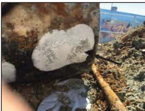
Photograph 5: The third UST was found in poor condition with a 4-inch diameter hole.
