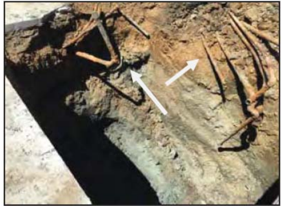
Photograph 14: Green staining was observed in the base and sidewalls of the fourth UST pit. Pipe lines were found running southwest towards the fifth UST and northwest into the subject property (arrows).
