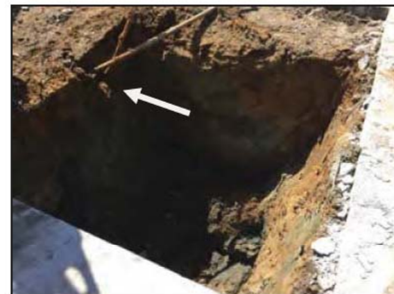
Photograph 6: Green staining was observed in the base and sidewalls of the third UST pit. Pipe lines were found running southwest towards the fourth UST (arrow).
