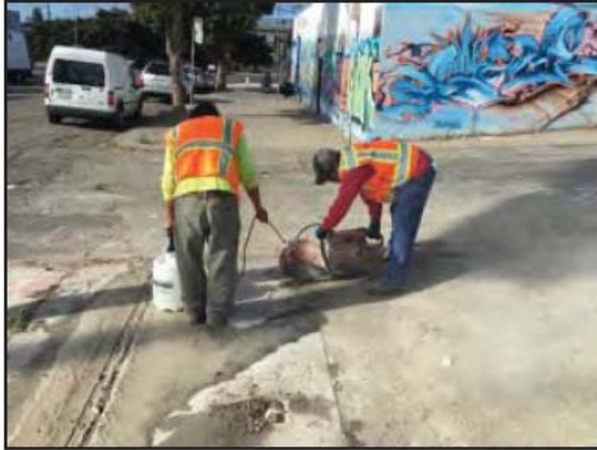
Photograph 19: A saw was used to cut the concrete slab above the fifth UST. The excavation area had previously been cleared for utilities by USA.
