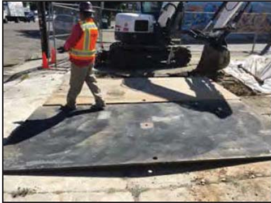
Photograph 7: Trench plates were placed over the open pits for safety until they were backfilled.
