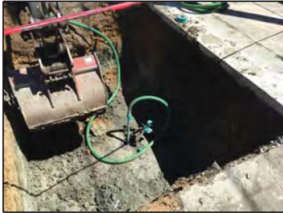
Photograph 21: The tank contents were pumped just before adding dry ice to the fifth UST.
