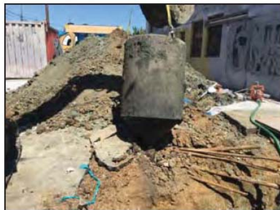
Photograph 11: The fourth UST was removed using the excavator bucket and was found to be an upright, conical tank.
