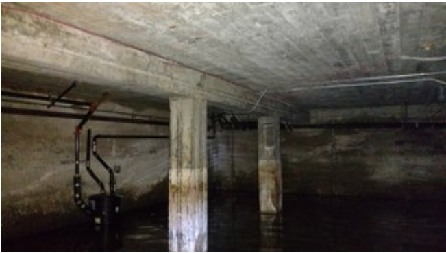
Photograph No. 16 – Northwest view of interior basement showing holding reservoir or pumping station located along west foundation wall of building (WGE, 3/1/17).
