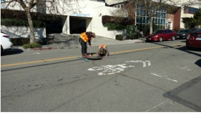
Photograph No. 9 – Northwest view from sidewalk of Webster Street site frontage showing Subtronic Corporation assessing depth and flow direction of sanitary sewer main during subsurface utility survey activities (WGE, 3/1/17).
